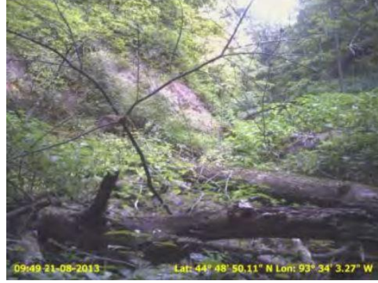
Unstable channel bottom and fallen trees cause toe of slope erosion and slope failure
