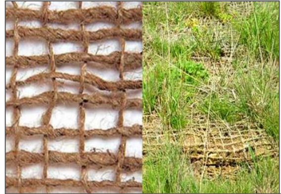
Image 2- 58: Jute ESC Blanket. After seeding the area and surface packing, the Jute blanket was installed. The grasses have germinated and grown through the loose weave (photo: CA DOT).
