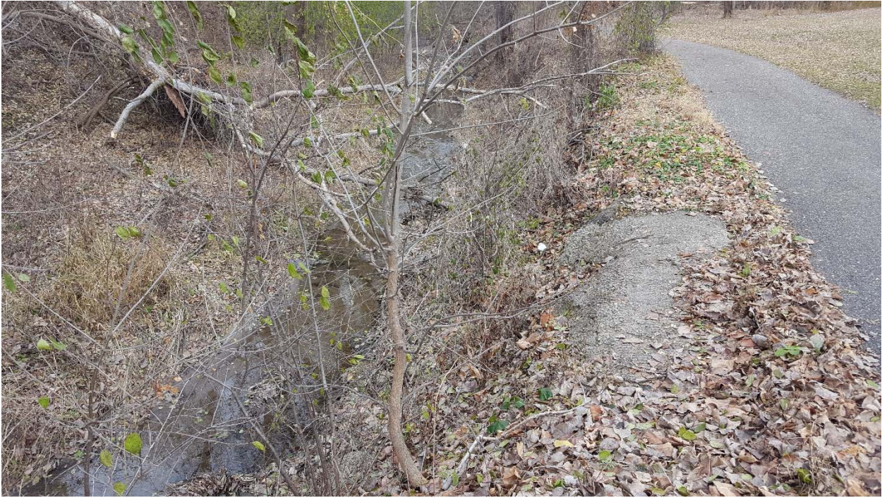
Photo 14: Site S3 – eroding bank between channel and paved trail near Lenzen Chevrolet
