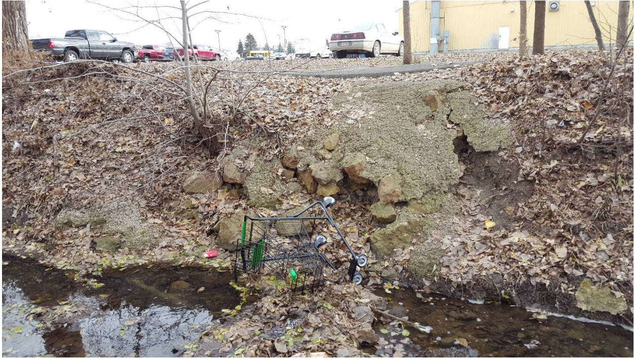
Photo 15: Site S4 – eroding bank and debris in the channel
