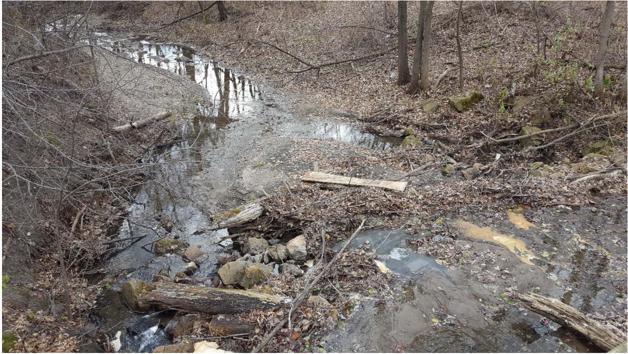
Photo 12: Site S1 – scour hole and erosion downstream of Crosstown Boulevard
