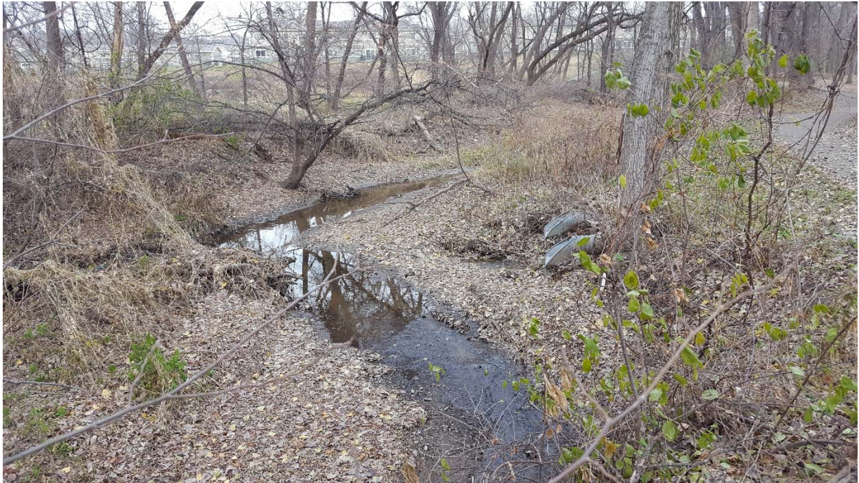
Photo 1: Site M2 –erosion around culvert outfalls.
