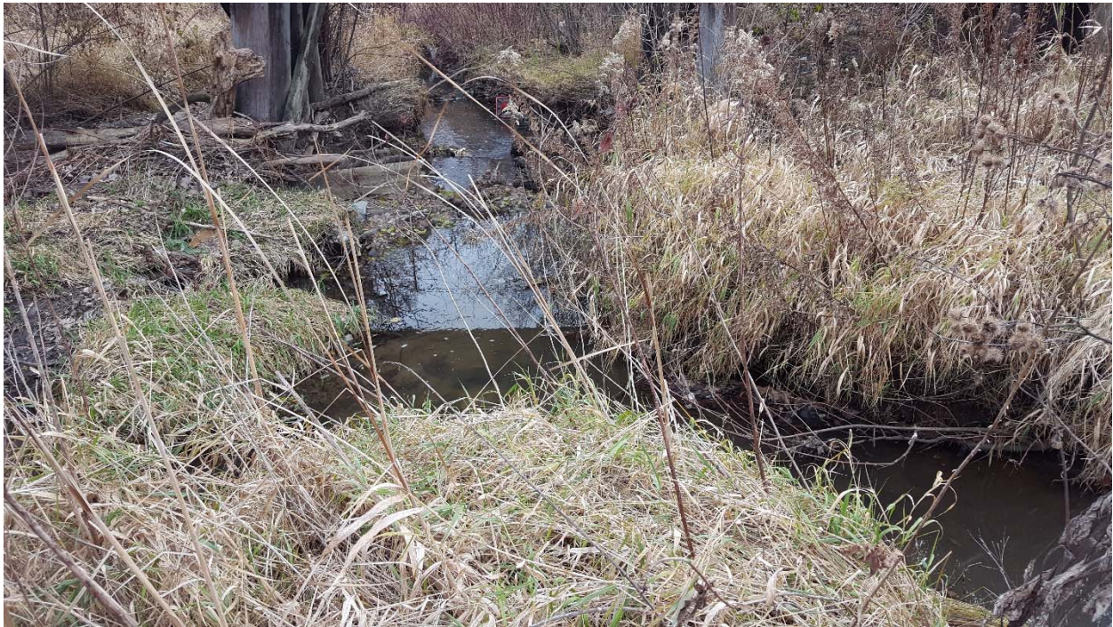
Photo 18: Site S8 – Two small headcuts in the channel between Chaska Boulevard and the old railroad bridge
