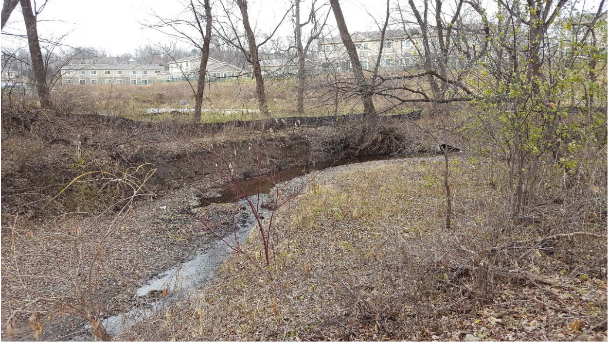
Photo 15: Site S5 – eroding bank and undercut trees
