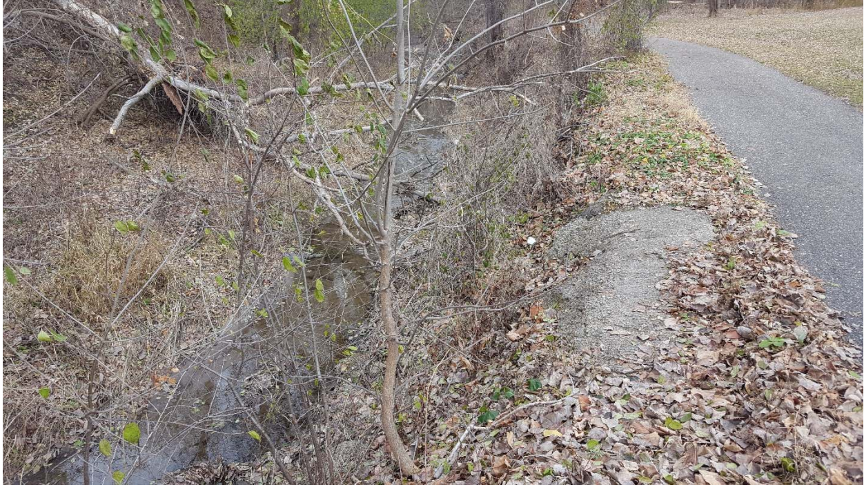
Photo 13: Site S3 – eroding bank between channel and paved trail near Lenzen Chevrolet
