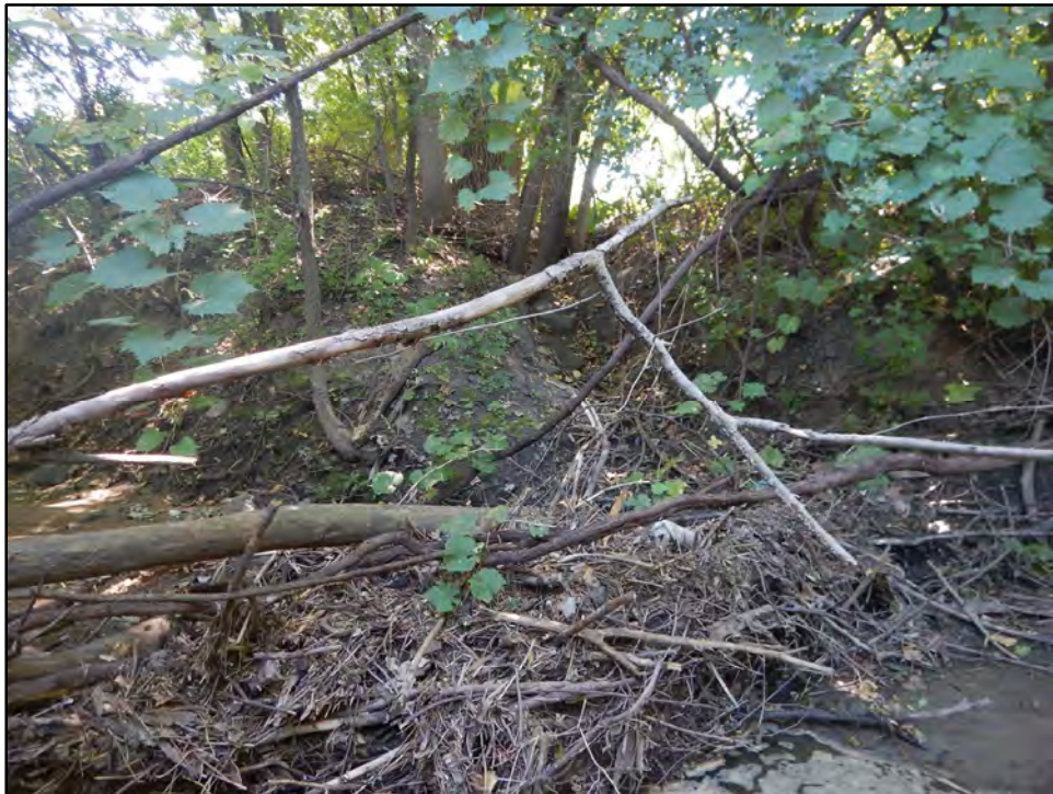
Photograph A-10: View east of debris.
