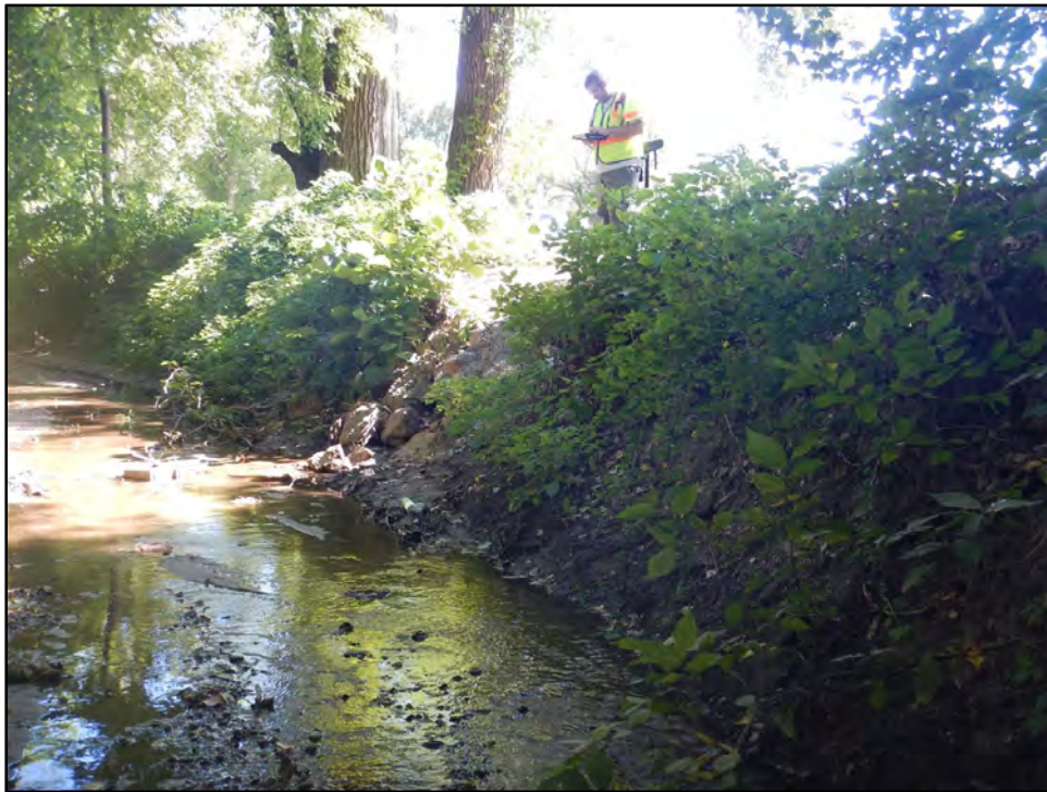
Photograph B-13: View north of eroded bank.
