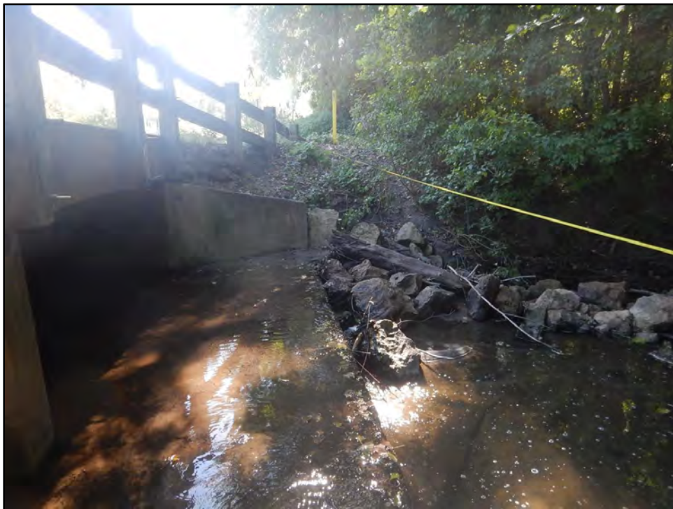
Photograph B-6: View southwest of bridge crossing and scour hole.
