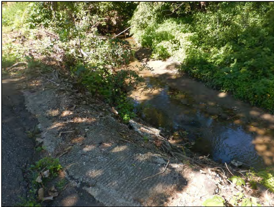
Photograph B-11: View south of eroded bank.
