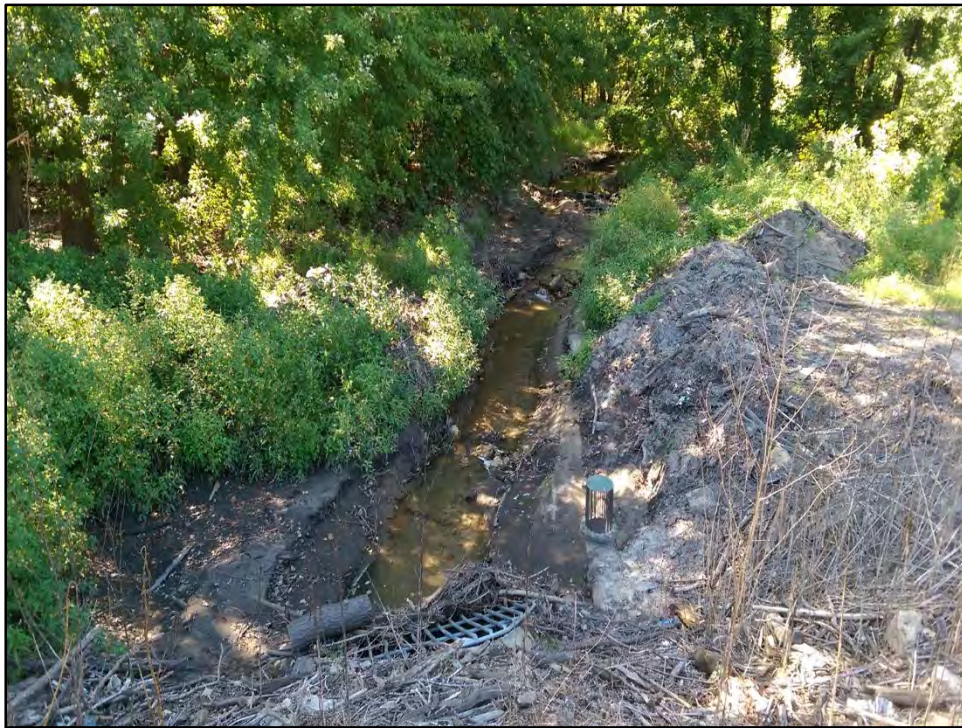
Photograph A-15: View west of debris and RCP.
