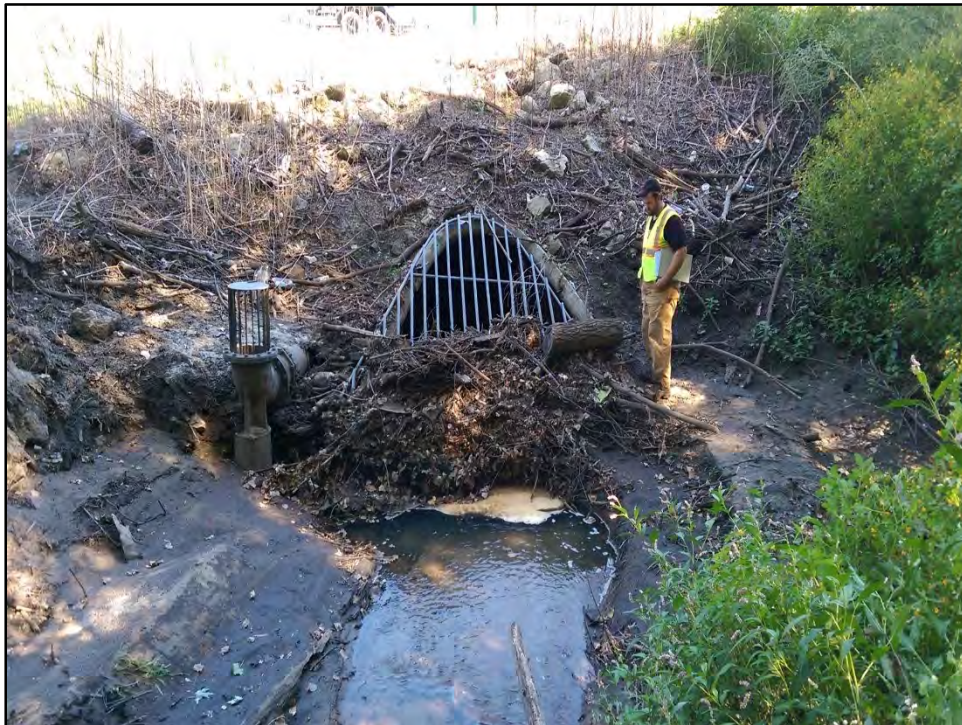
Photograph A-14: View east of debris at RCP.
