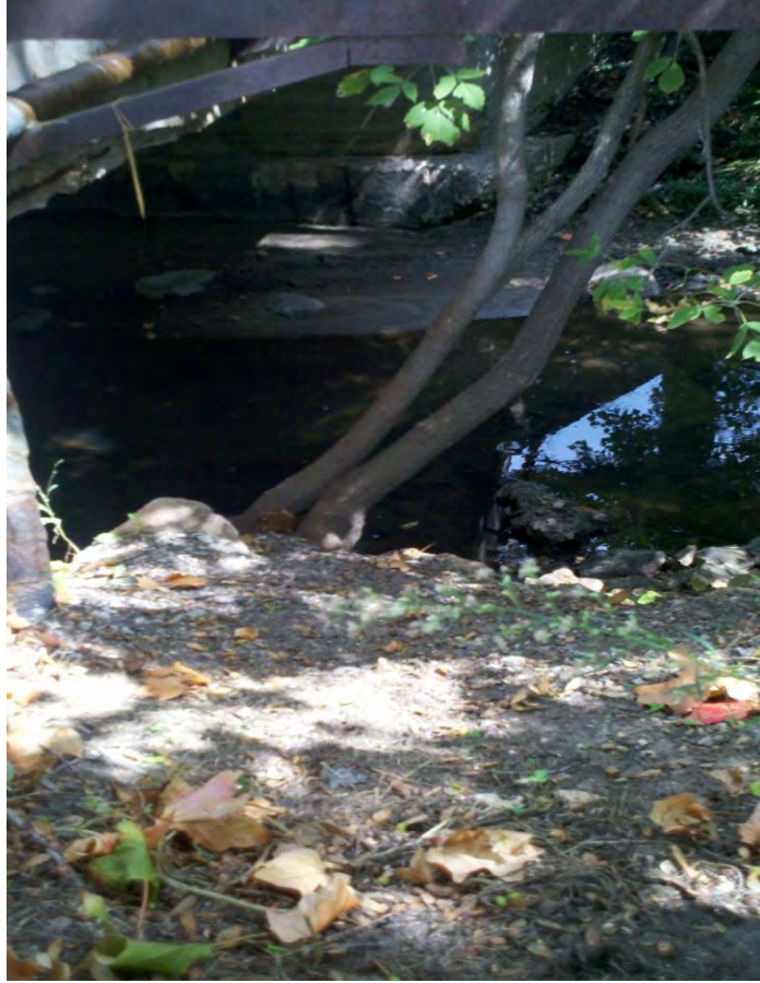
Photo 14. Downstream of bridge near intersection of Oak St and E. Sixth St., East Chaska Creek
