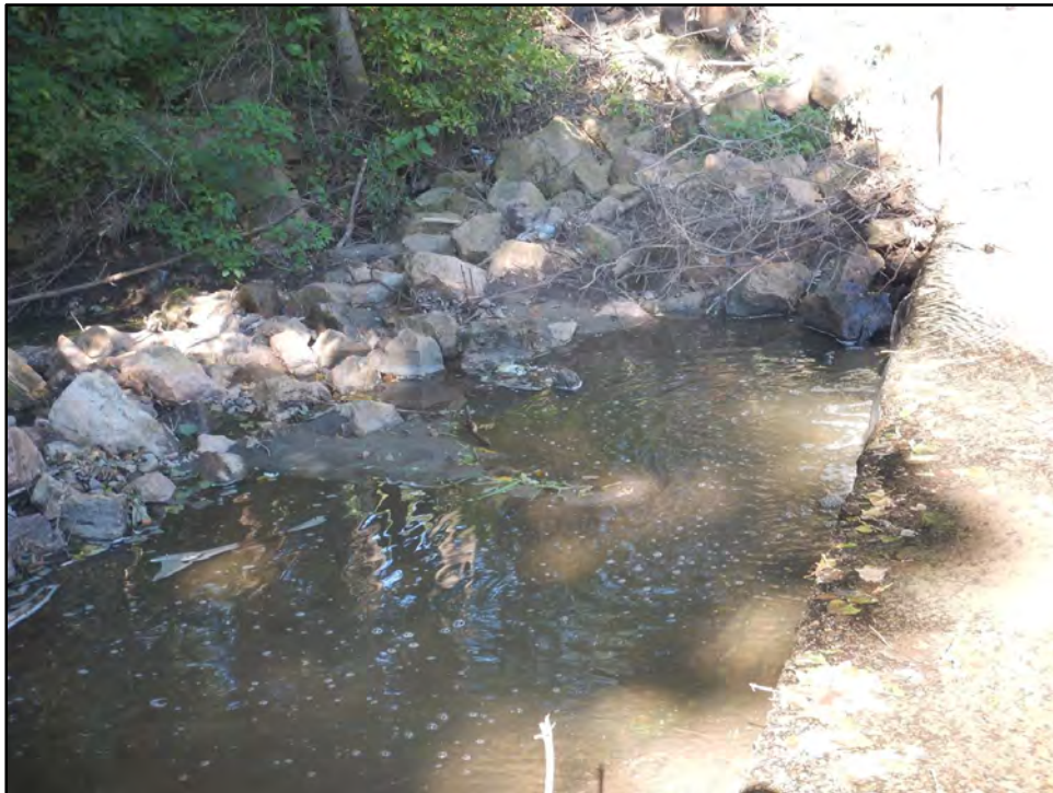
Photograph B-1: View northwest of scour hole.
