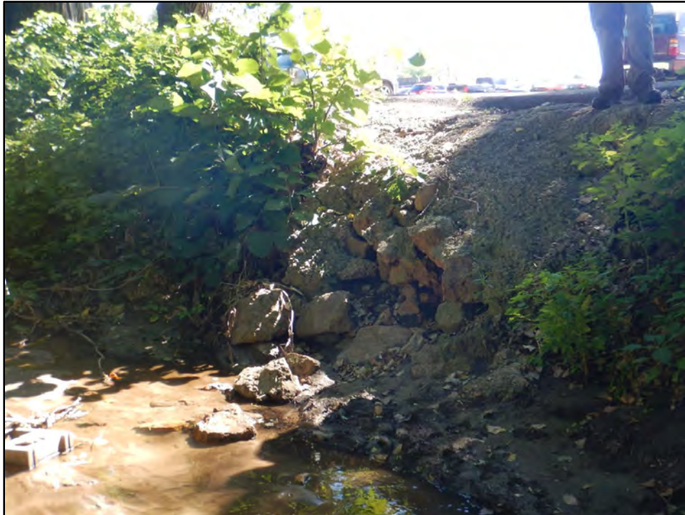
Photograph B-10: View east of bank erosion.
