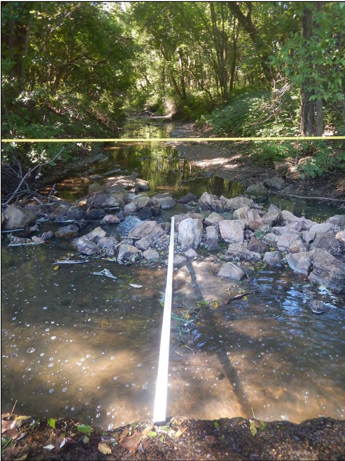
Photograph B-4: View southwest of scour hole.
