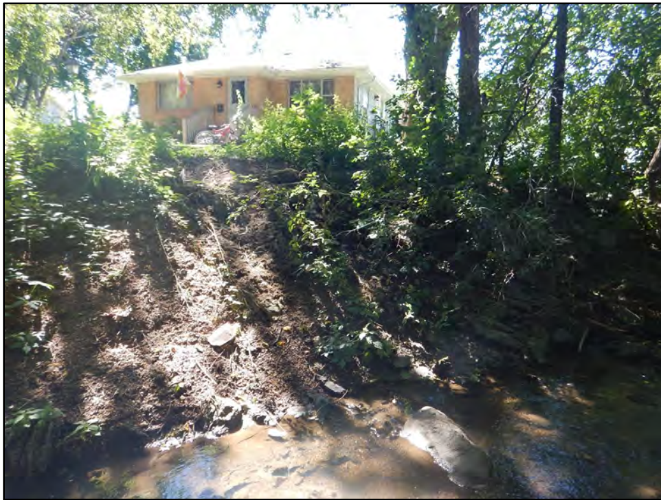
Photograph B-15: View south of eroded bank.
