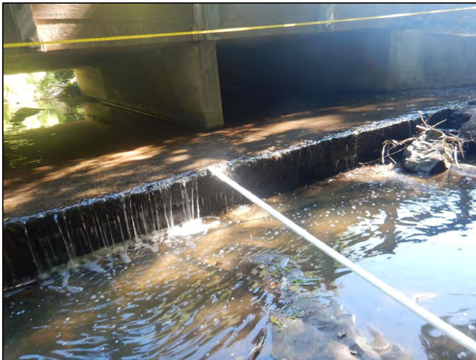
Photograph B-8: View north of bridge crossing and scour hole.
