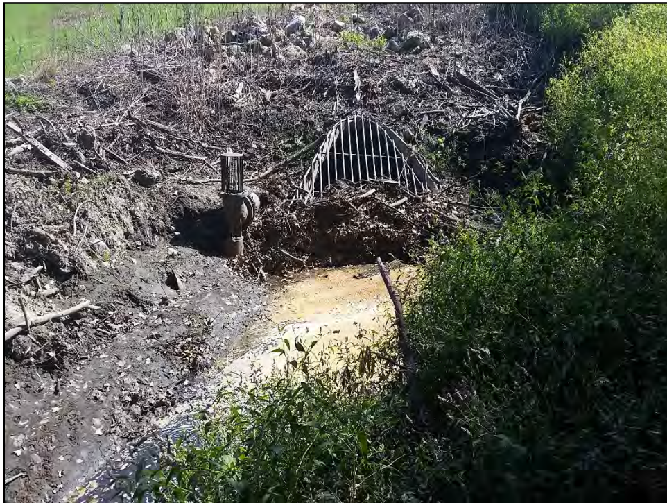
Photograph C-9: View east of foam at levee from potential sanitary/septic source.
