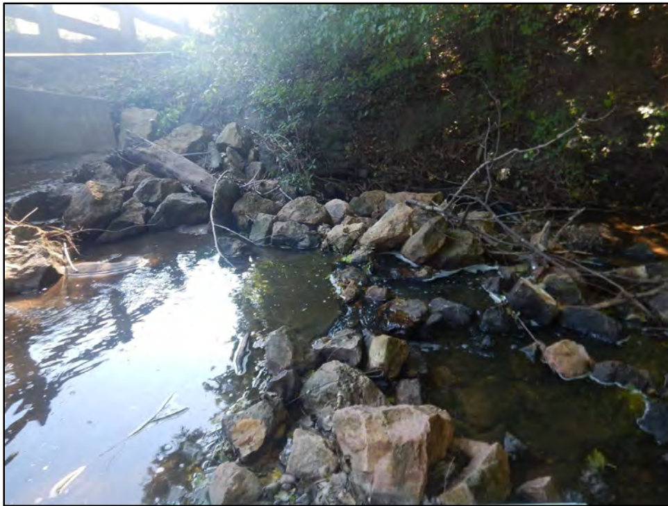
Photograph B-7: View southwest of debris and scour hole.
