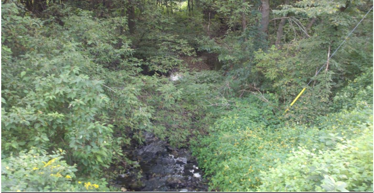
Photo 7. East Chaska Creek riprap effectively dissipating stream velocity (Downstream of Engler Blvd)
