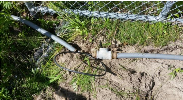
Sensor line damage and repair, 2016
