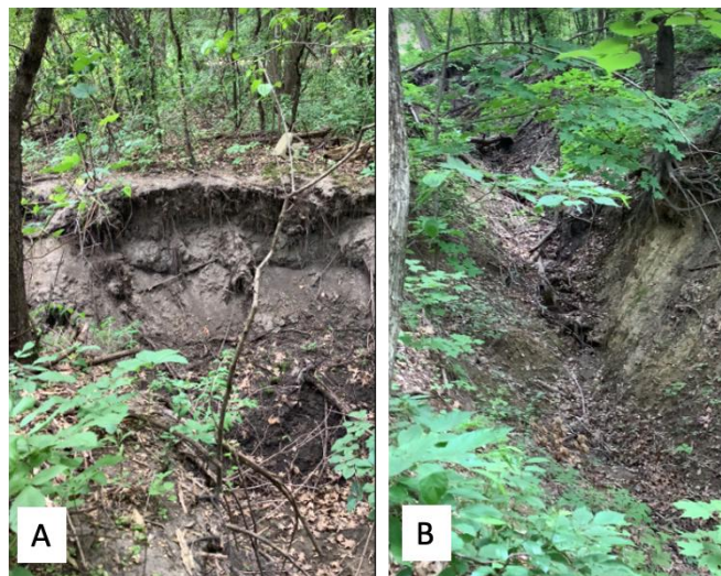
Figure 23. Photos of CHH11. A) Headcut viewed from gully bottom. B) V-shaped banks viewed from gully bottom.
