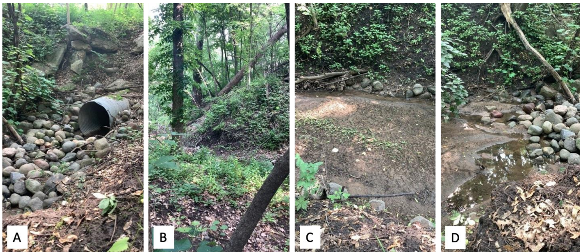
Figure 8. Photos of gully BVL62. A) Headcut with large pipe outfall and surrounding rip rap. B) Facing North at bank from the side of the headcut. C) Gully bottom condition. D) Image of water pooling at bottom of rip rap
