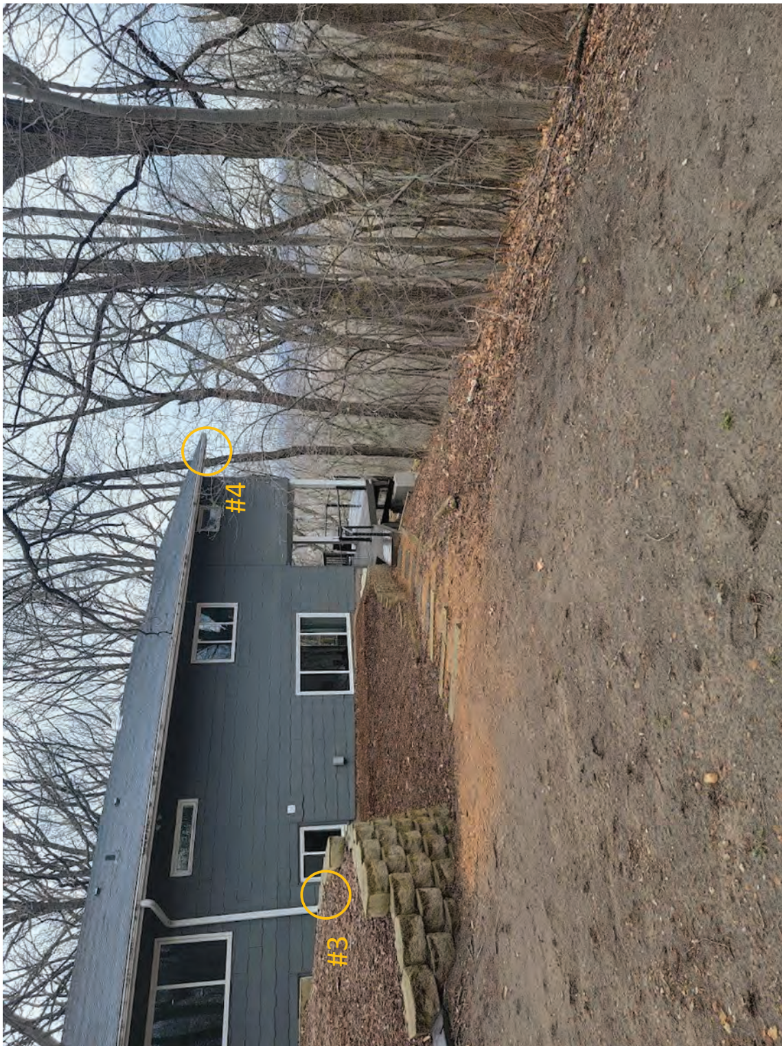
535 Lakota Lane – west side of house (discharge points circled in yellow)
