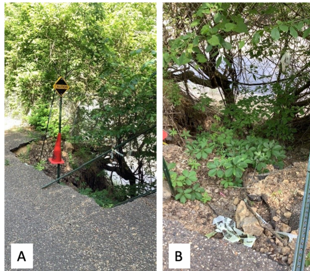
Figure 21. Photos of SHK16. A) Gully marked with sign as it encroaches on paved trail. B) Looking down at the gully from the headcut.
