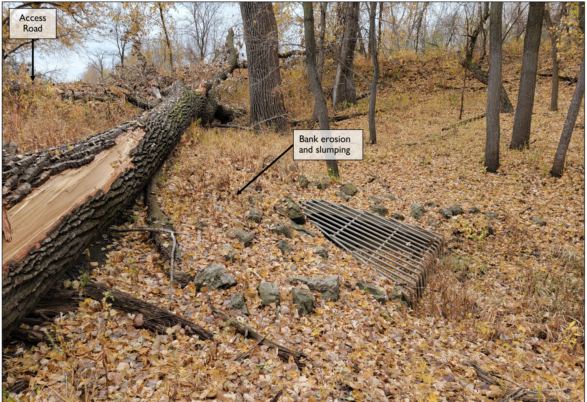
4. Looking west at downstream embankment, culvert outfall apron and trash guard, and left bank.
