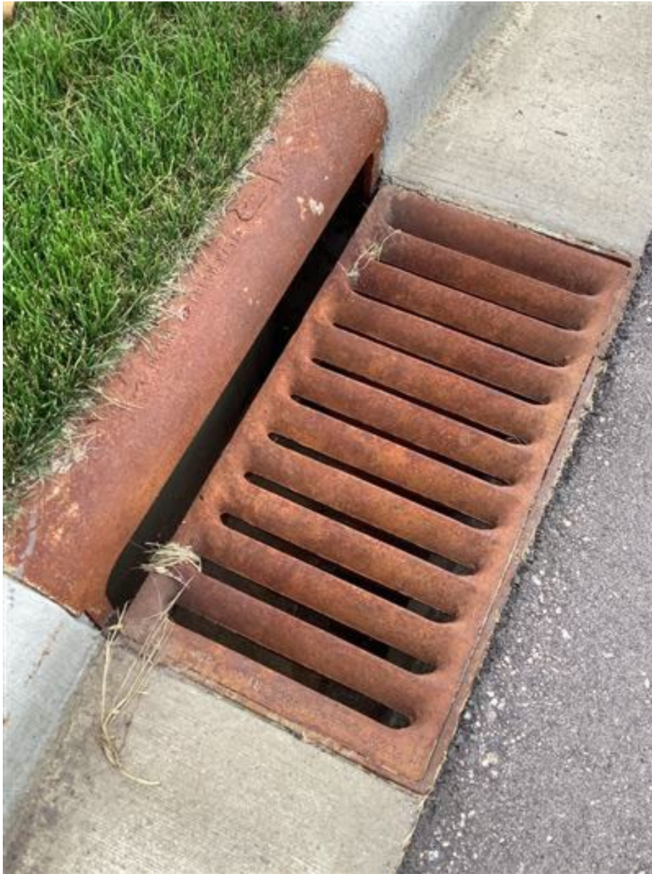
Figure 4. All inlets are free of protection and have no sediments
