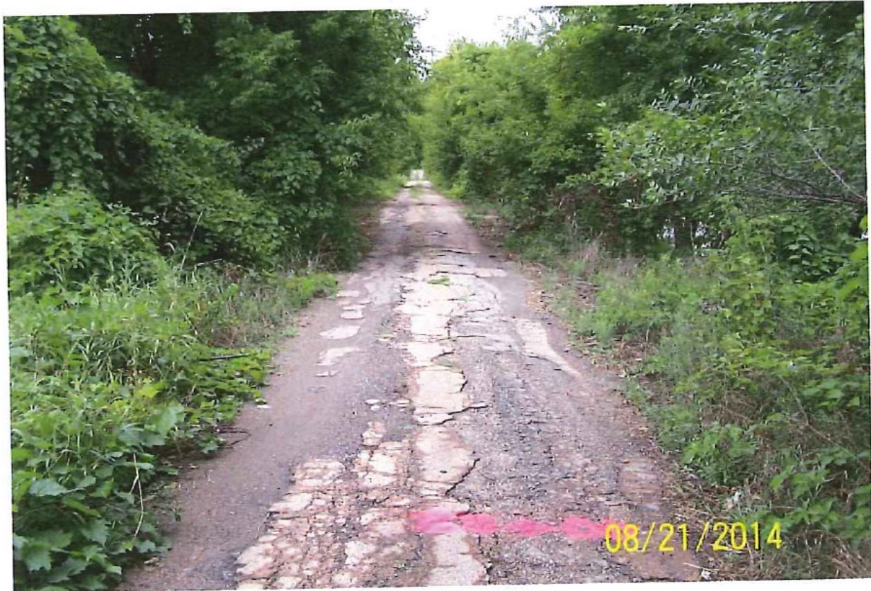
Figure 3. 2015 Vernon Avenue pavement condition (AET, 2015)
