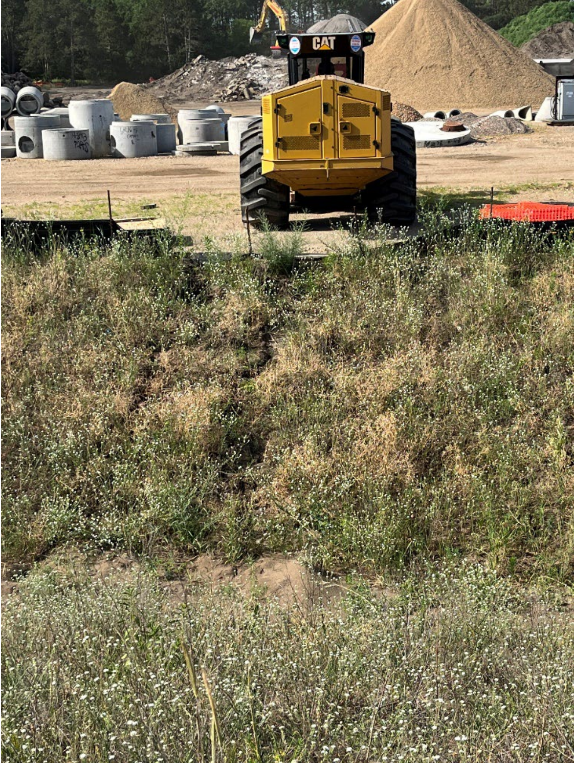
Figure 2. Rill formation in pond sidewall
