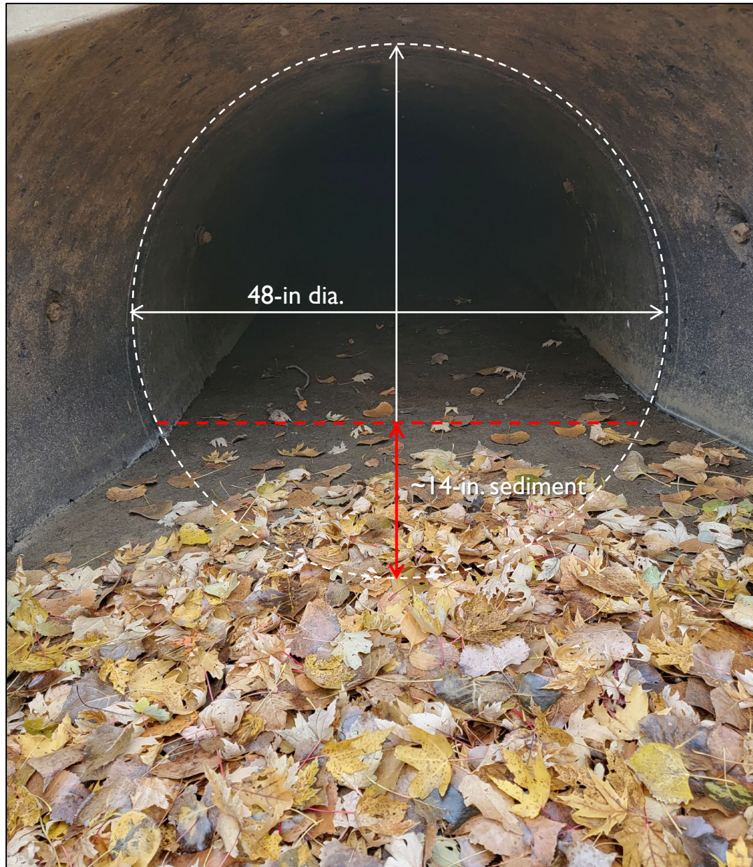
5. Looking upstream from the downstream culvert apron at pipe sedimentation (approximate culvert diameter shown with white dashed lines, approximate sedimentation shown in red).
