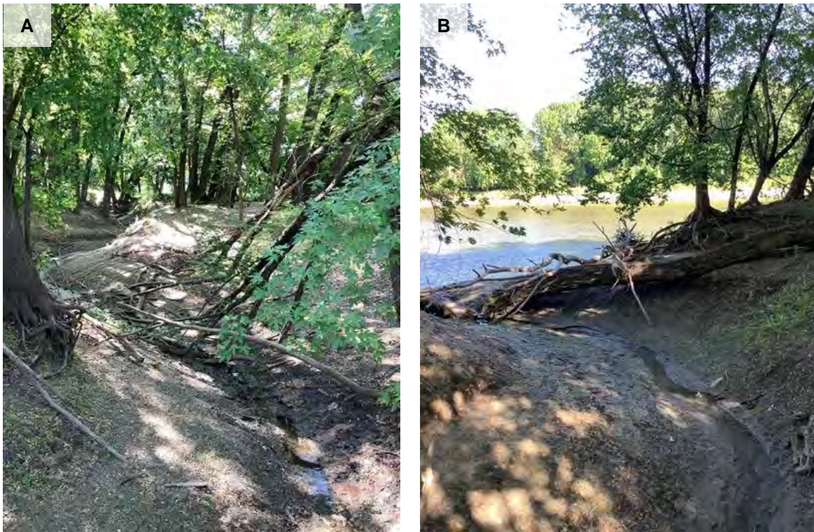
Figure 26. Photos of Gully 06:04-08:59. A) View upstream from the bridge crossing the gully. Exposed roots from trees on the right bank are visible along with some broken branches lying in the middle of the gully. B) View of the gully's confluence with the MN River, where there is visible severe degradation on the lower banks right near the stream.
