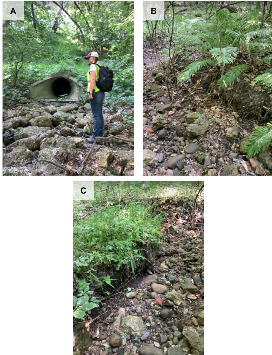
Figure 8: Photos of Gully 06:23-09:48 A). Looking upstream at pipe outfall, B) Looking downstream at right bank, C) Looking downstream at gully channel
