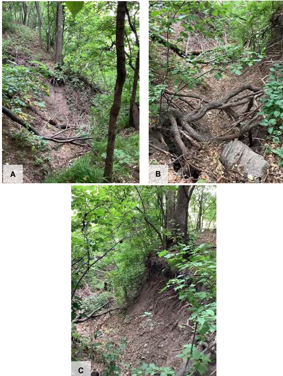
Figure 11: Photos of Gully 07:21-11:43 A) Downstream view of left bank, B) Downstream view of gully middle, C) Downstream view of right bank
