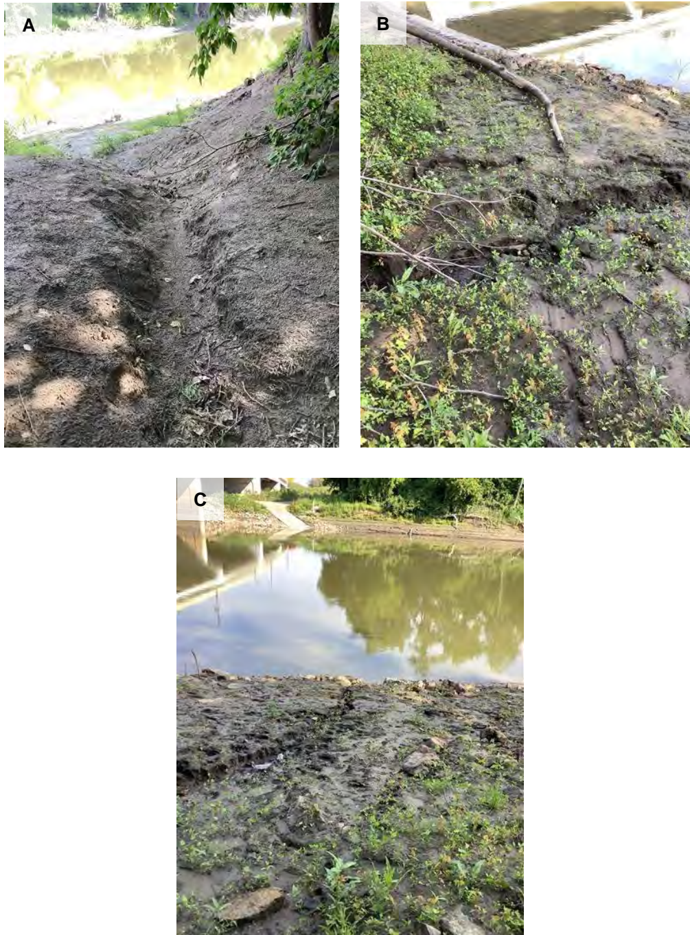
Figure 42: Photos of Gully 07:08-09:17. A) Downstream view of the gully, B) Downstream view showing the severely eroding left bank of the gully, C) Downstream view of the gully's confluence with the Minnesota River
