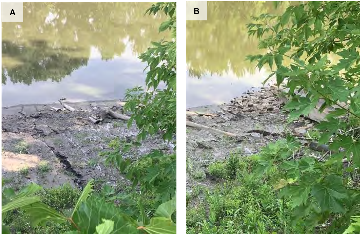
Figure 43: Photos of Gully 07:08–09:29. A) Downstream view of mini gullies and broken pipe. There was a very steep drop-off along with a lot of vegetation, so pictures were difficult to obtain. B) Downstream view of where pipe outfall broke and now drains
