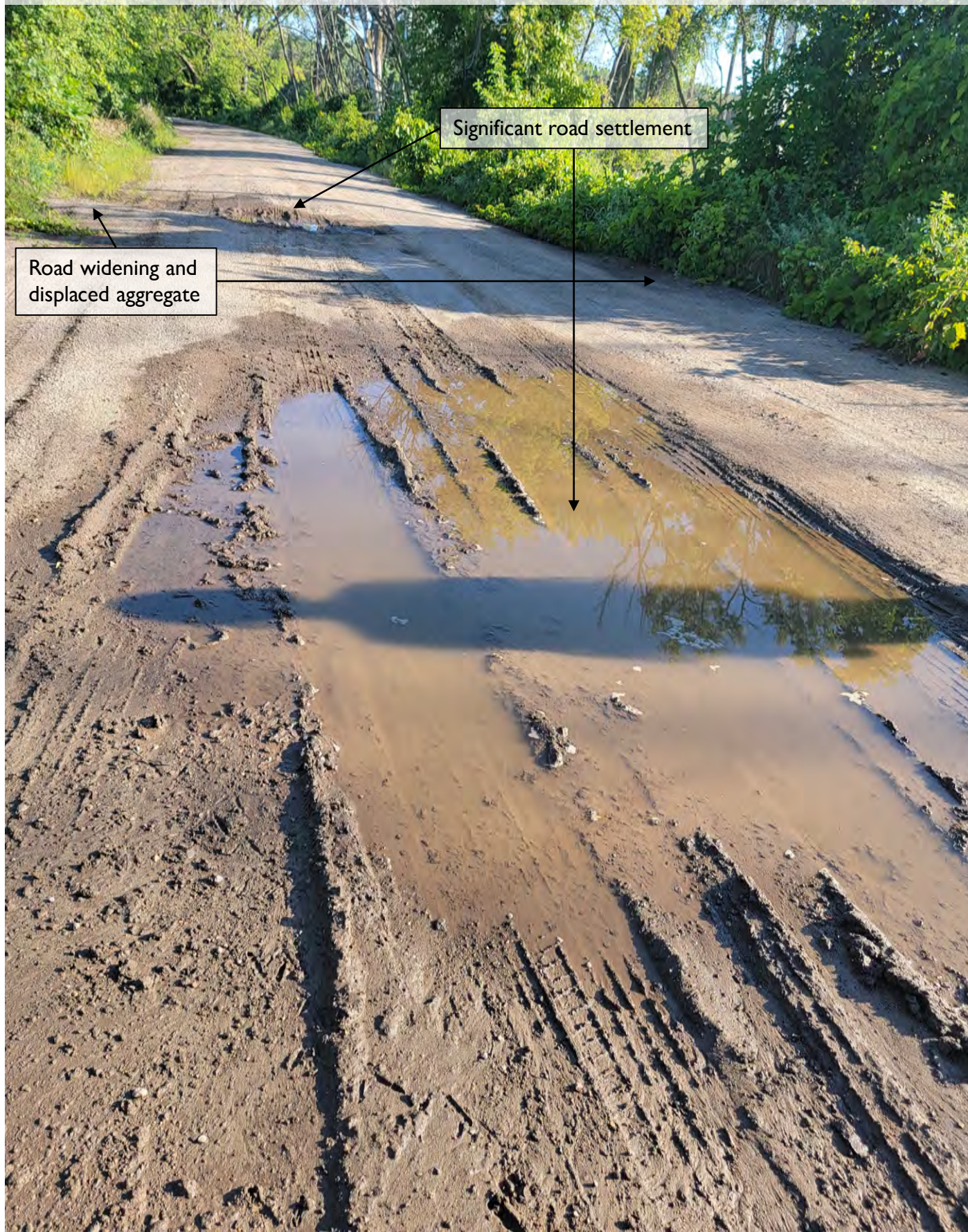
Photo 4A. Vernon Avenue settlement and rutting, looking north
