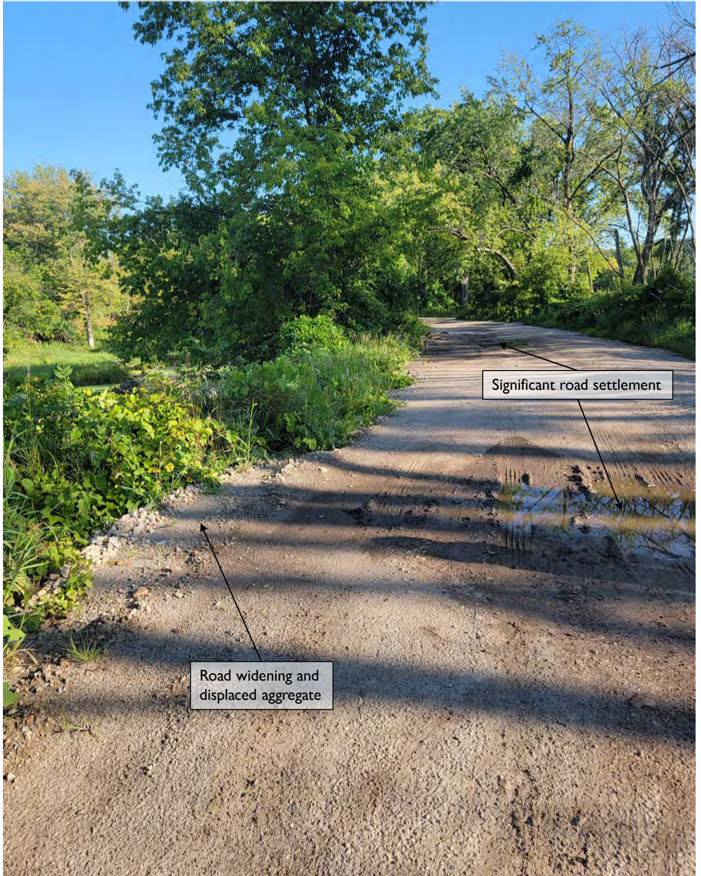
Photo 5. Vernon Avenue road widening and settlement, looking north
