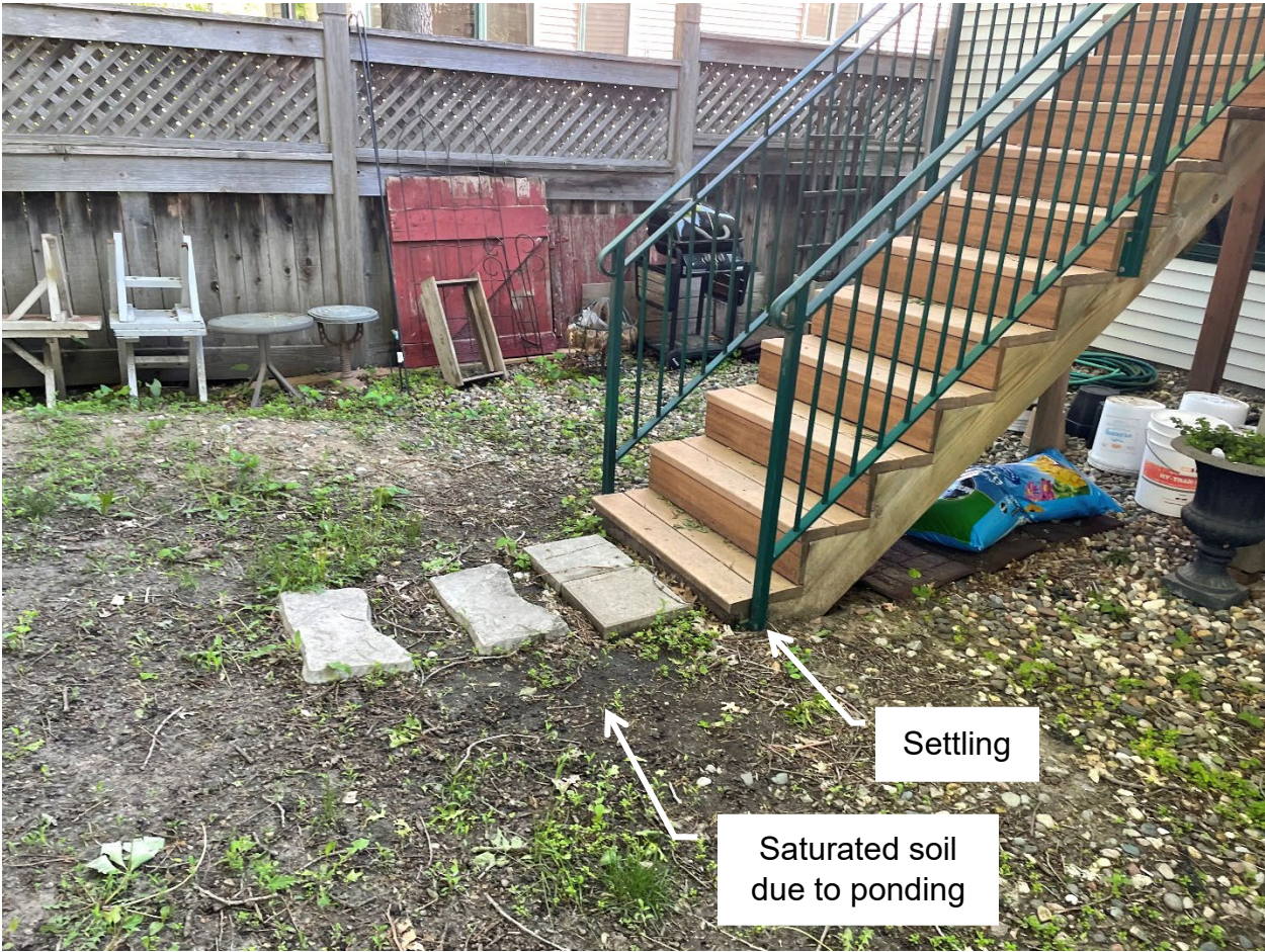
Figure 4. Settlement observed at deck stairs on June 2, 2022
