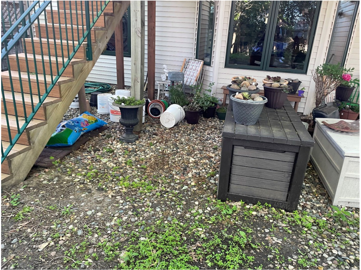
4. Location of ponding near the deck stairs and the foundation of the house (currently dry)
