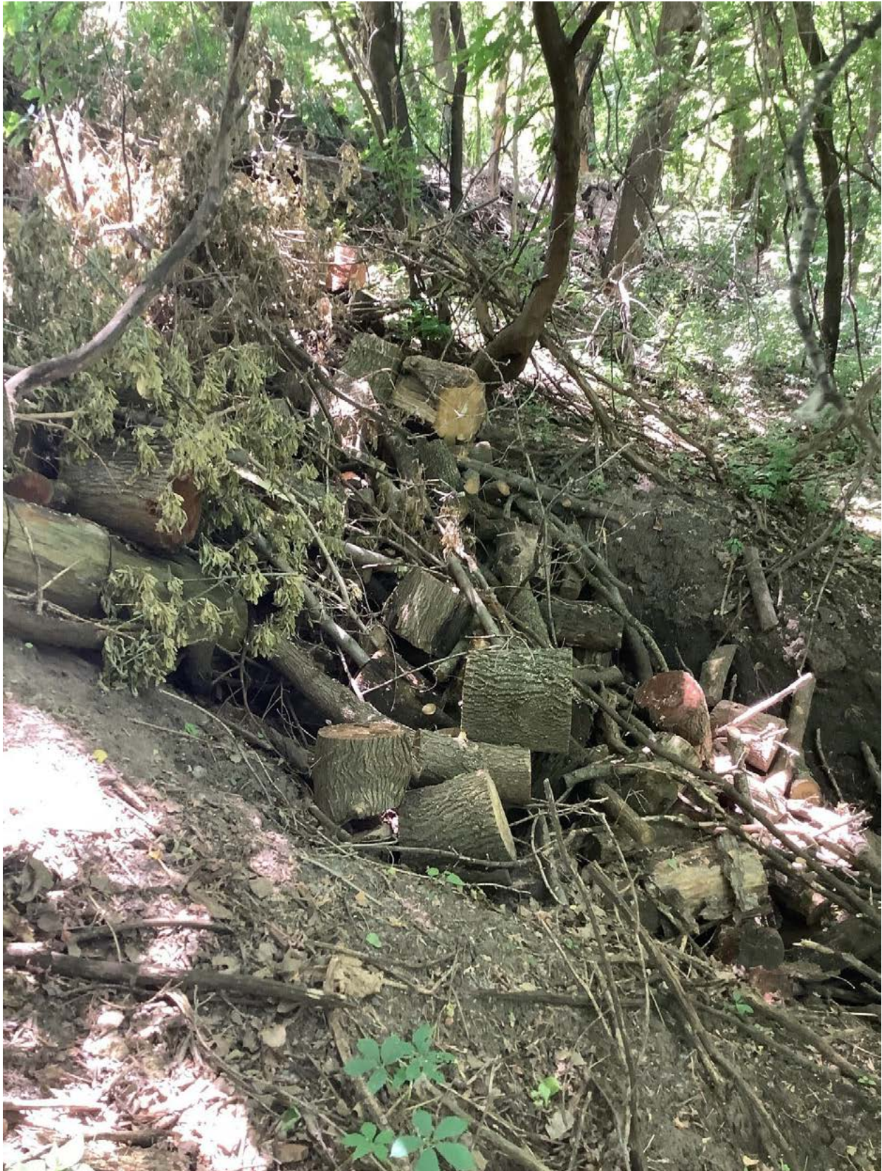
Figure 43. Gully stabilization attempt behind Wuthering Heights Road.
