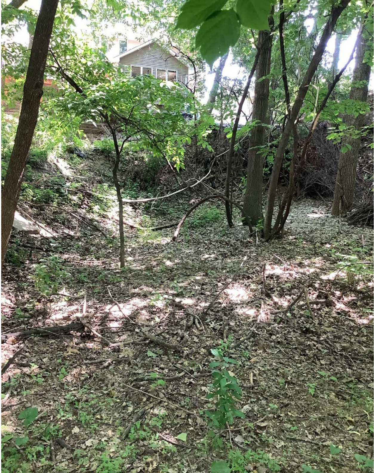
Figure 56. Gully erosion and sedimentation in upper Unnamed 4 watershed (behind 3101 Chandler Court).
