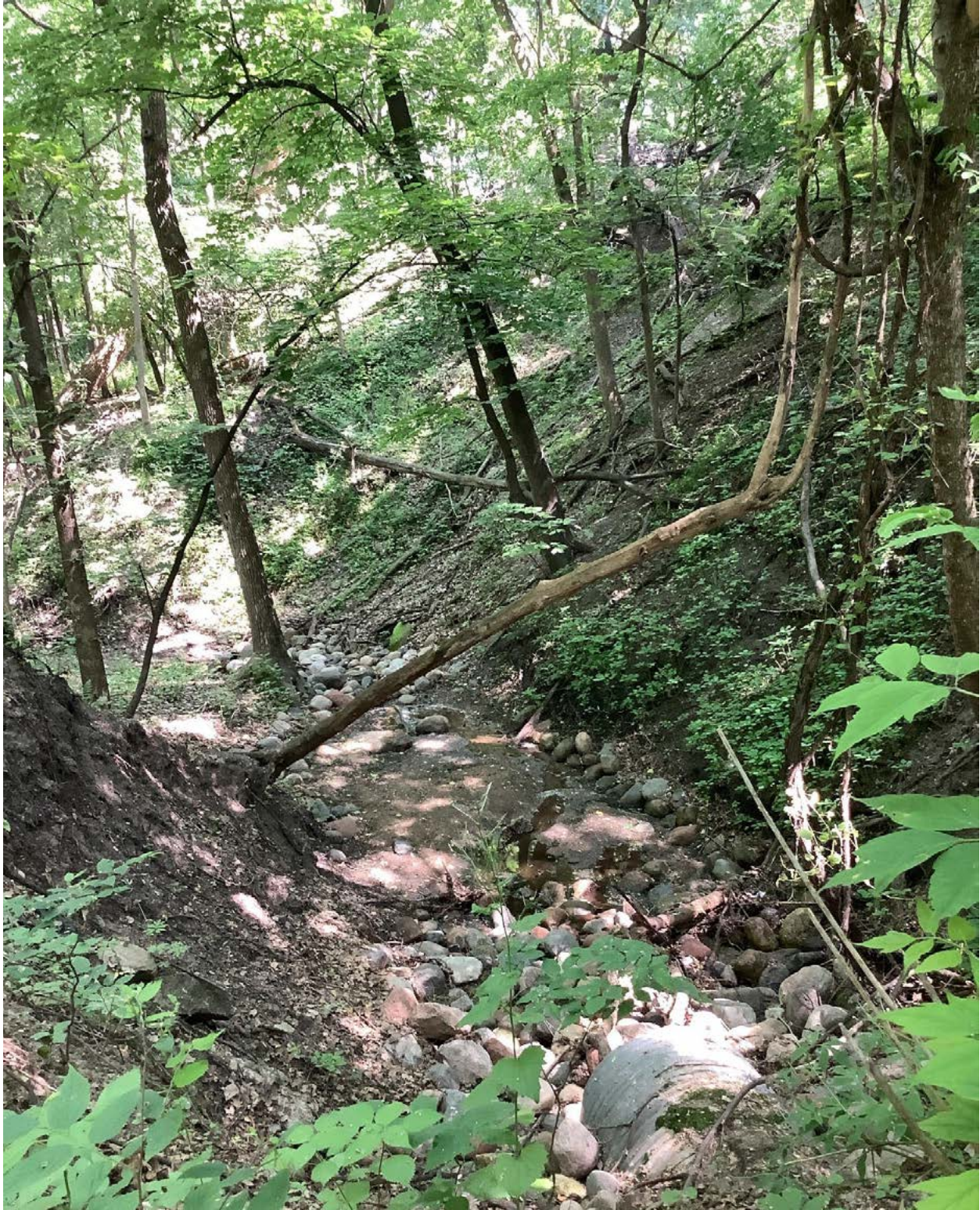
Figure 54. Gully erosion in upper Unnamed 4 watershed from stormwater outfall near 10805 Chatham Court.
