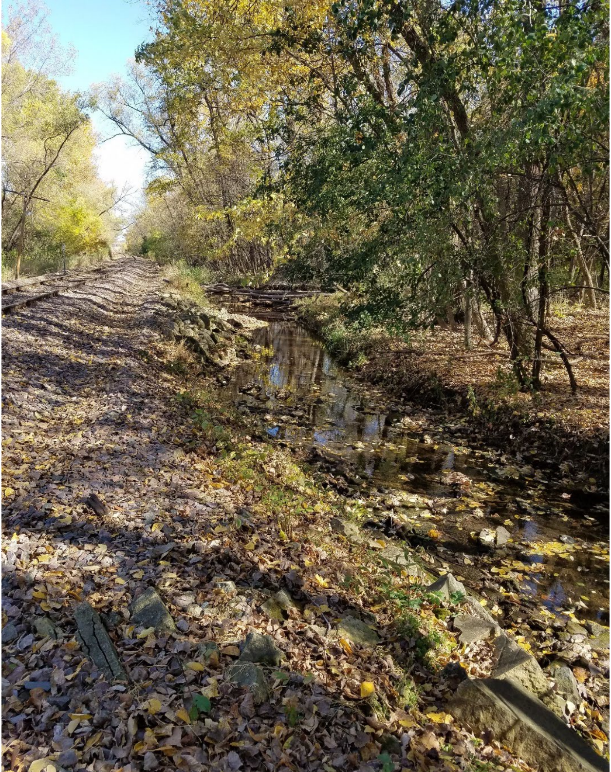
Figure 62. Union Pacific railbed armoring opposite stormwater outfall on October 13, 2020.
