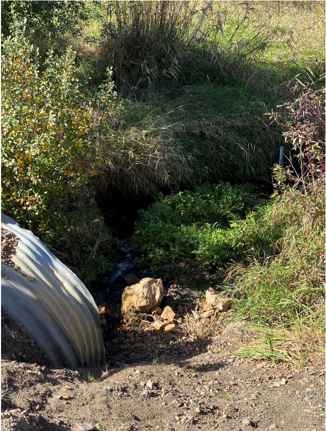
Figure 44. Kennaley's Creek downstream of the Union Pacific culvert, October 13, 2020.
