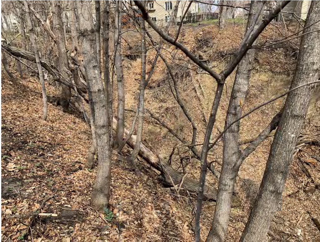
Concentrated discharges at top of slope causing slope erosion (STA 7+00)
