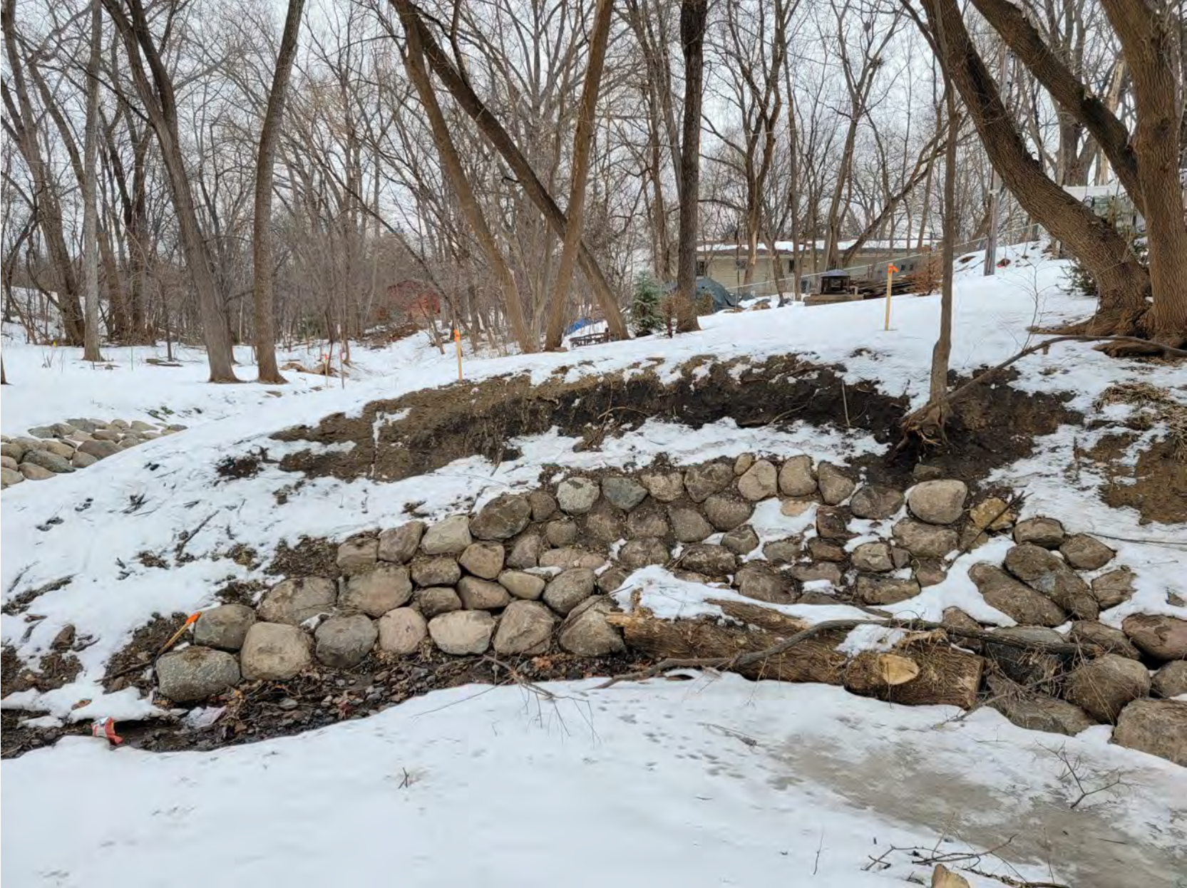
Looking across at anchored slope protection on right bank downstream from gabions (log, rock, grading, and hydroseed)
