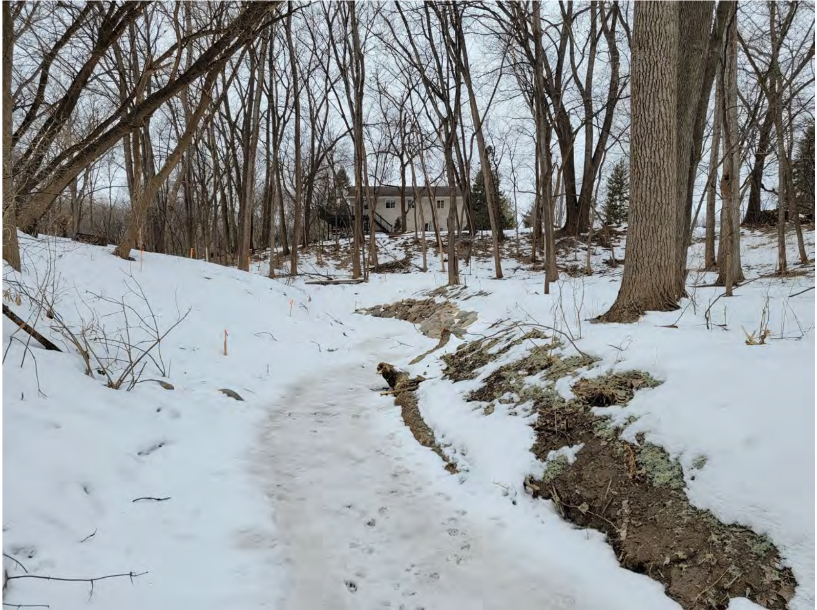
Looking downstream near end of construction with anchored slope protection on right bank using large logs and rock. Rock ditch check was not visible due to recent snow cover.
