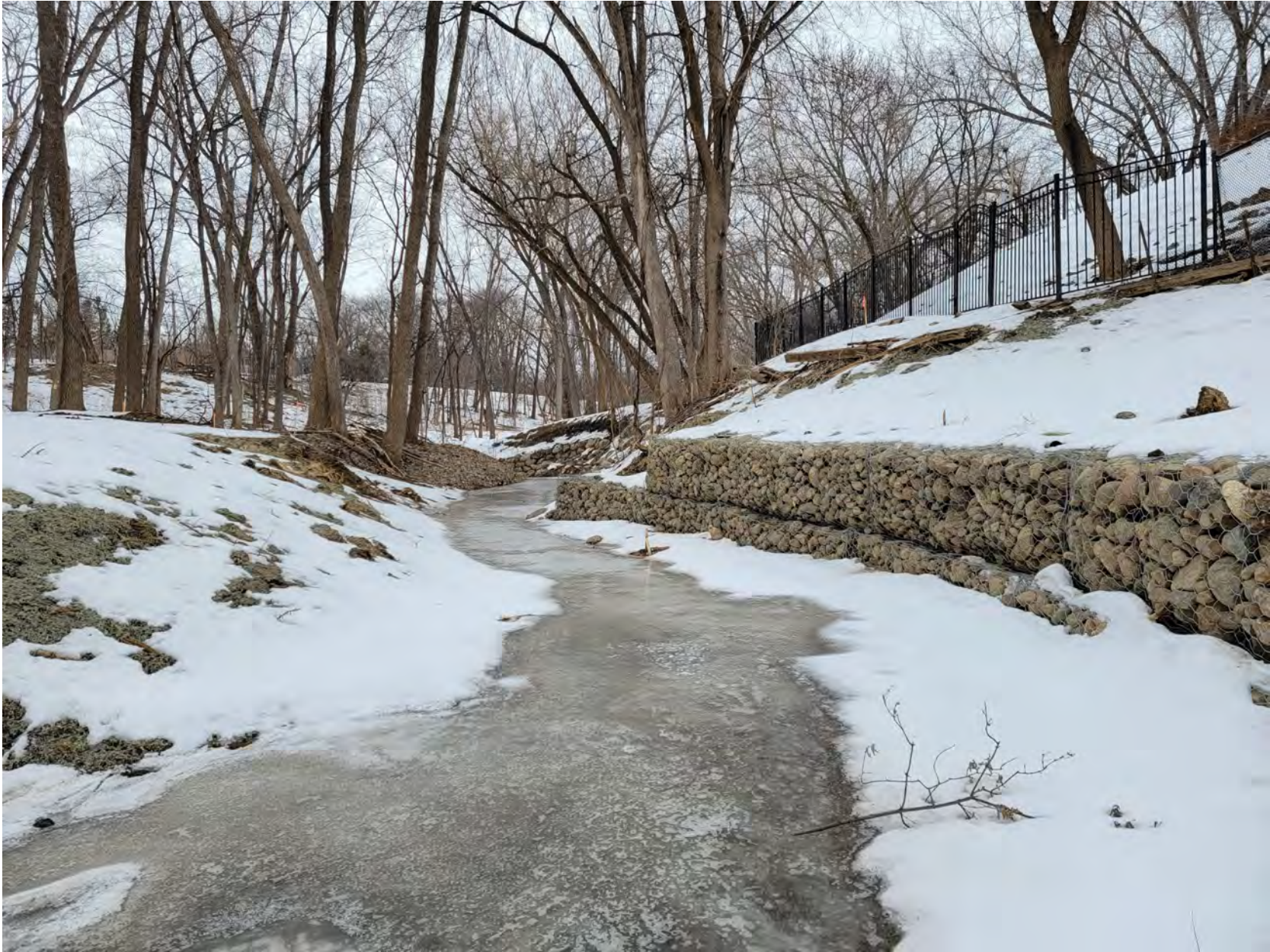
Looking downstream in channel at left bank anchored slope protection (grading and hydroseed) and gabion wall on right bank
