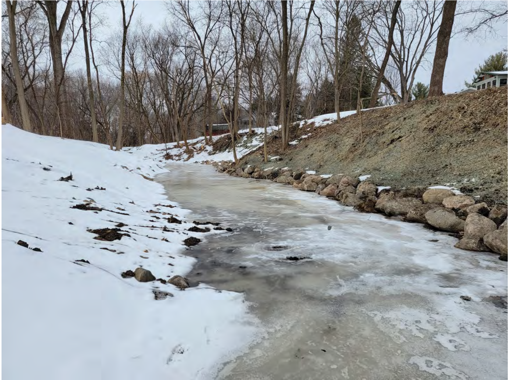
Looking upstream from channel at Glenview Drive construction access point at right bank anchored slope stabilization (grading, hydroseed and rock toe)
