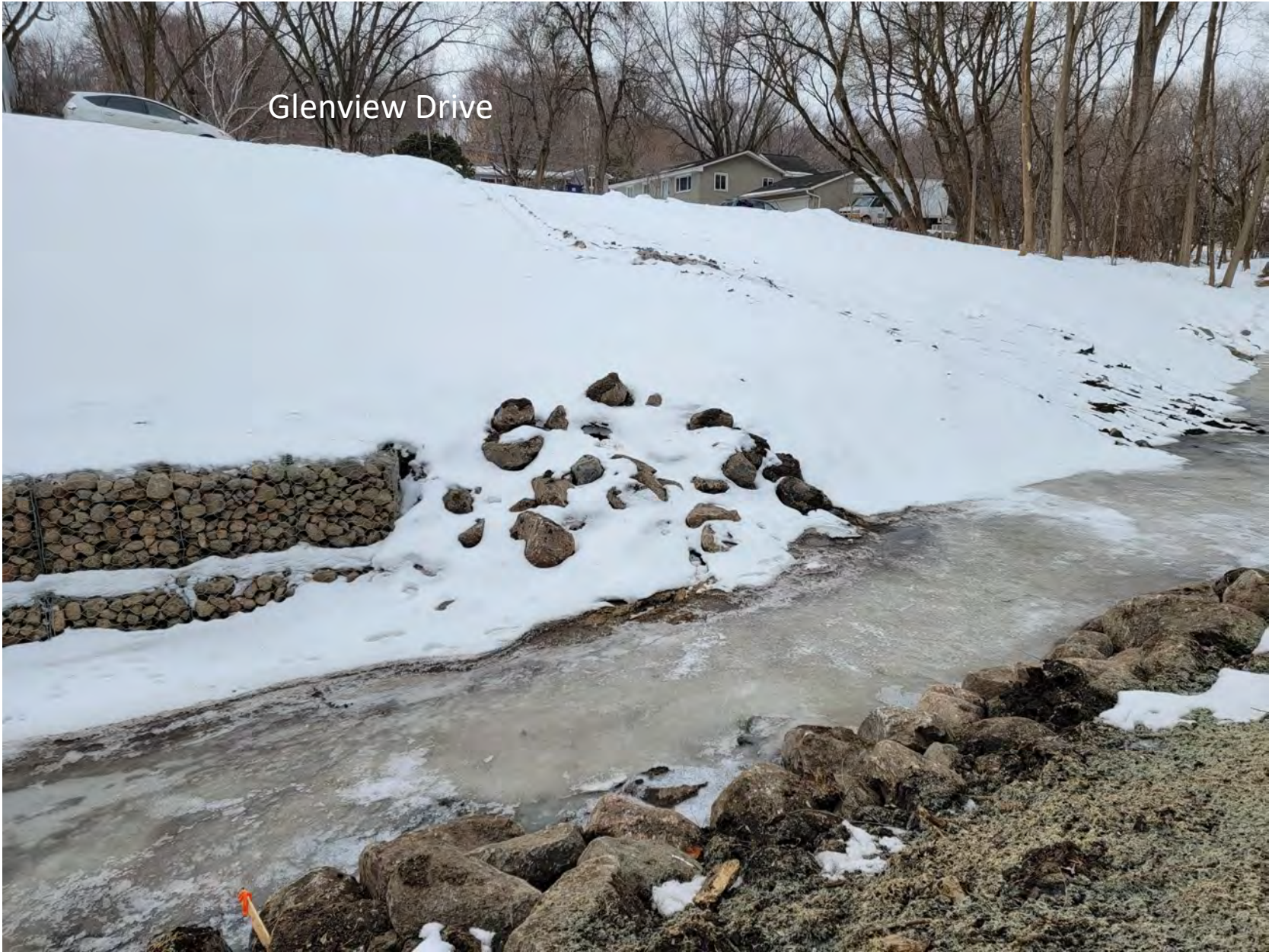
Looking upstream in channel at right bank gabions, riprap outfall, and Glenview Drive construction access
