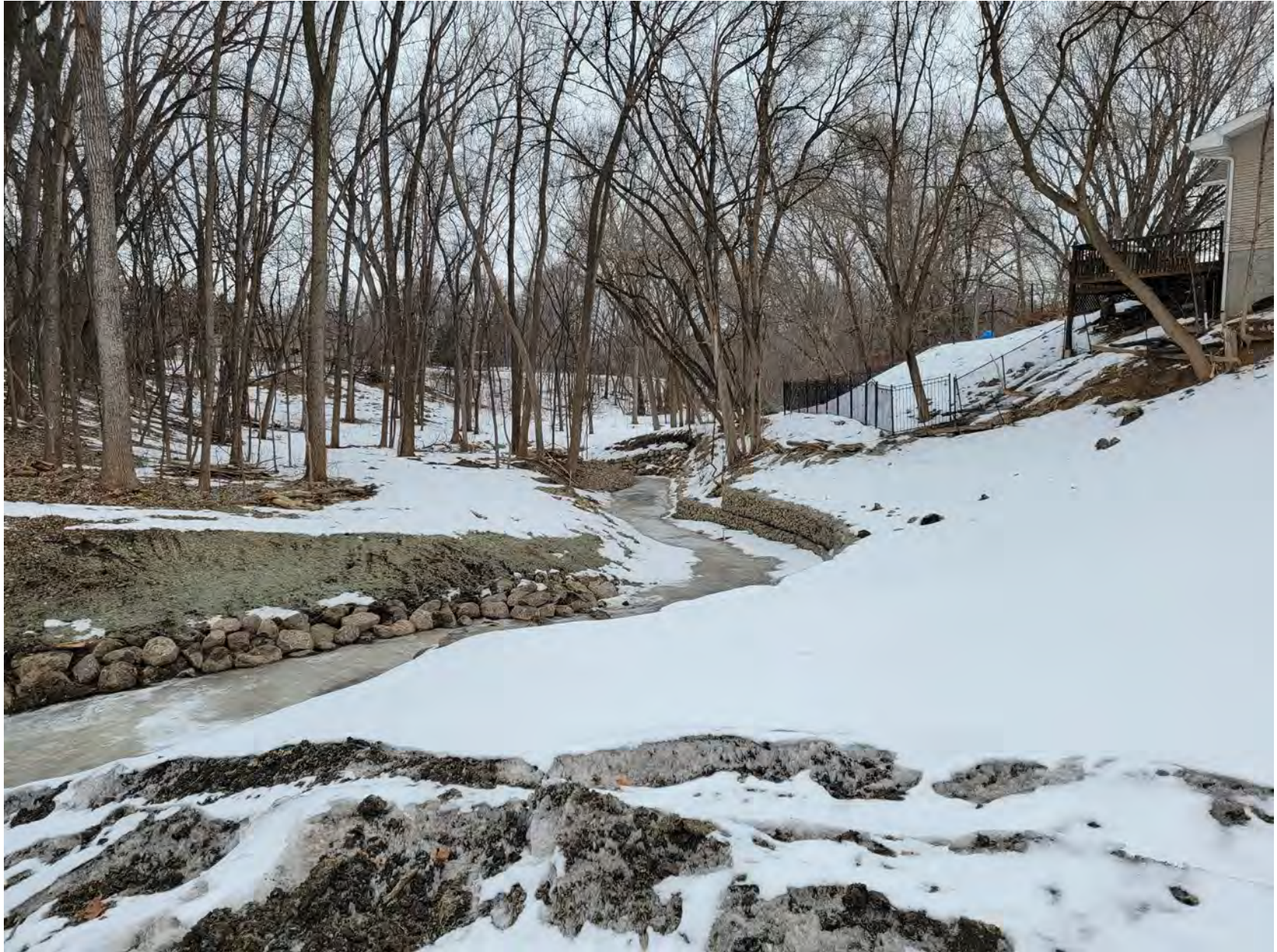
Looking downstream from Glenview Drive construction access point. Anchored slope protection with rock toe on left bank and gabion wall on right bank
