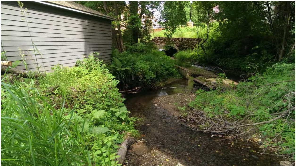
Photo 8: Downstream section of stream with significant erosion encroaching on the garage and damaged retaining wall
