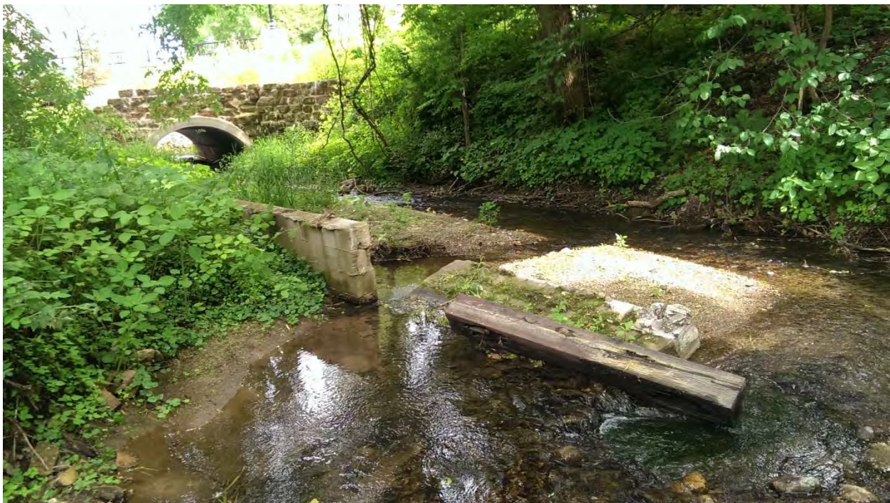
Photo 10: Close-up of damaged retaining wall most likely caused by stream path change
