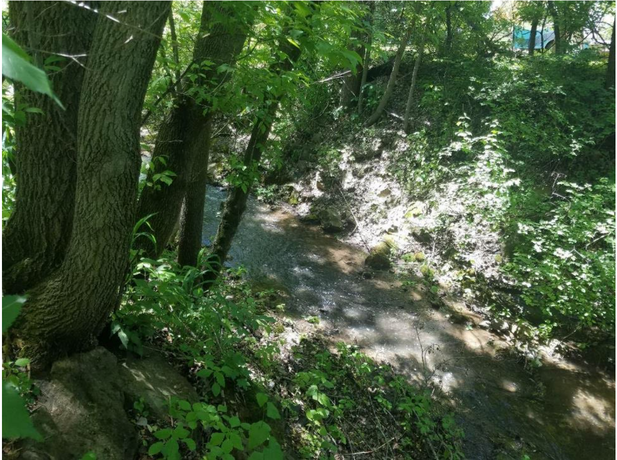
Figure 11. Spring Creek looking downstream from 112 5th Street (Site 1); note the near-vertical left bank and pistol-butted trees, indicating slow slope movement; erosion and slope instability are also present on the opposite right bank.
