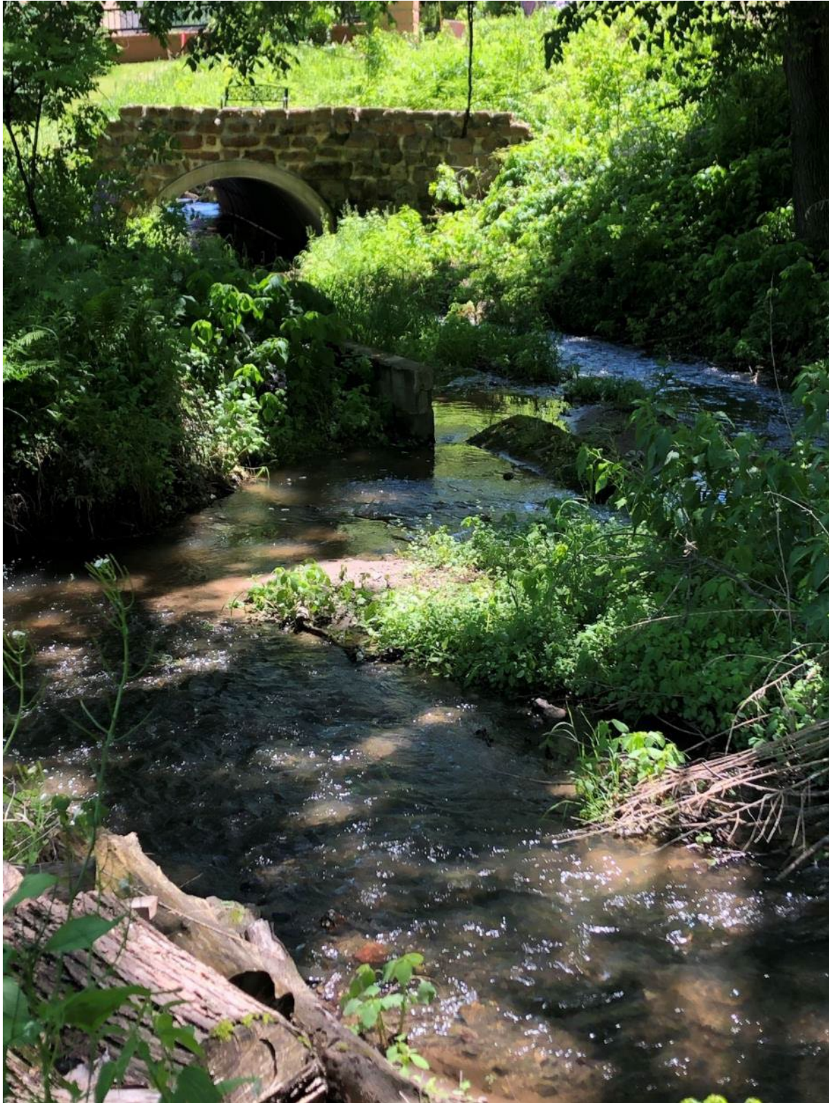
Figure 19. Spring Creek looking downstream at a failed retaining wall in the channel.
