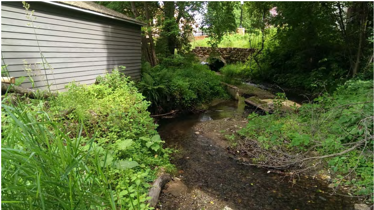
Photo 8: Downstream section of stream with significant erosion encroaching on the garage and damaged retaining wall
