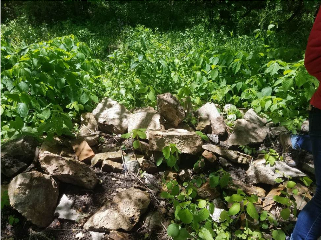
Figure 14. Riprap and debris placed on left bank at 420 and 416 Broadway.
