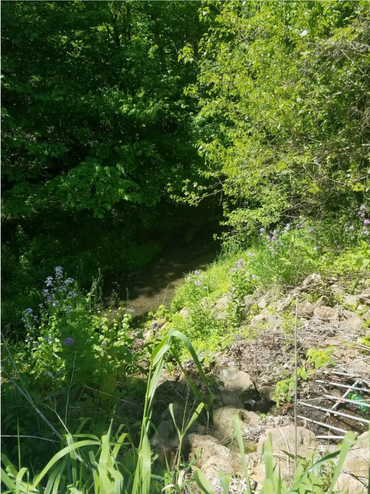
Figure 13. Looking upstream at riprap bank protection and stormwater outfall at the end of 5th Street West.
