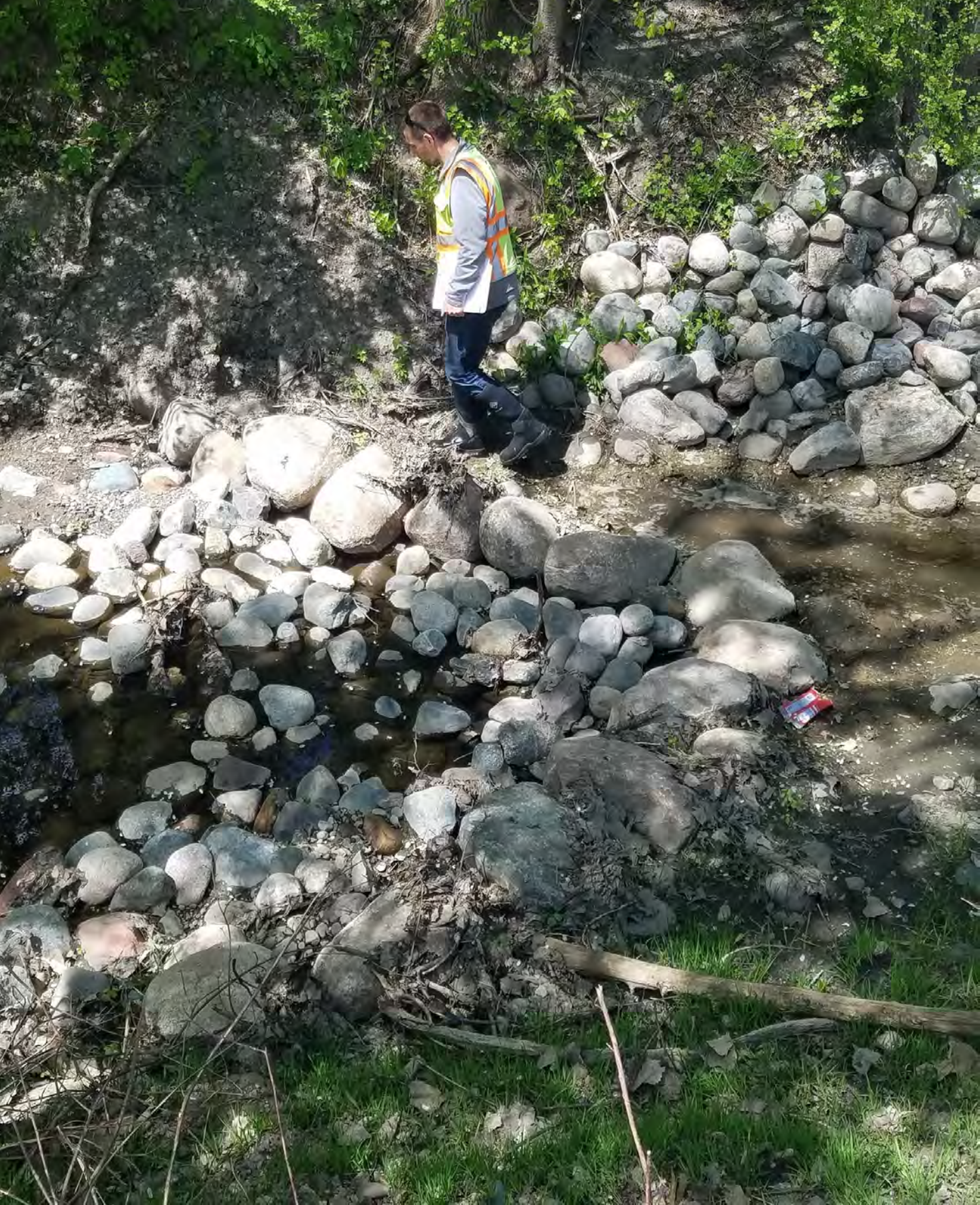
Photo Location #4: Example of right bank erosion at cross vane.
