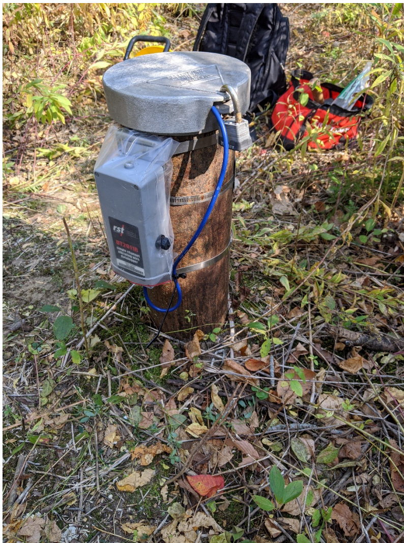
Photo 3: Well SB-6 with vibrating wire piezometer cable (blue) and datalogger (grey) attached
