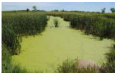
Renville County has approved a petition by County Ditch 77 landowners to extend this open channel in Limbo Creek for the Ditch 77 outlet, which is covered by sediment. Tom Cherveny / West Central Tribune file photo
