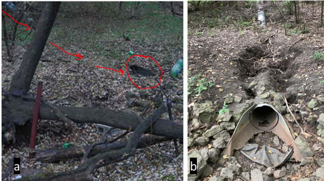
Figure 27. A comparison of the pipe outfall and gully head cut between 2008 (a) and 2020 (b).
