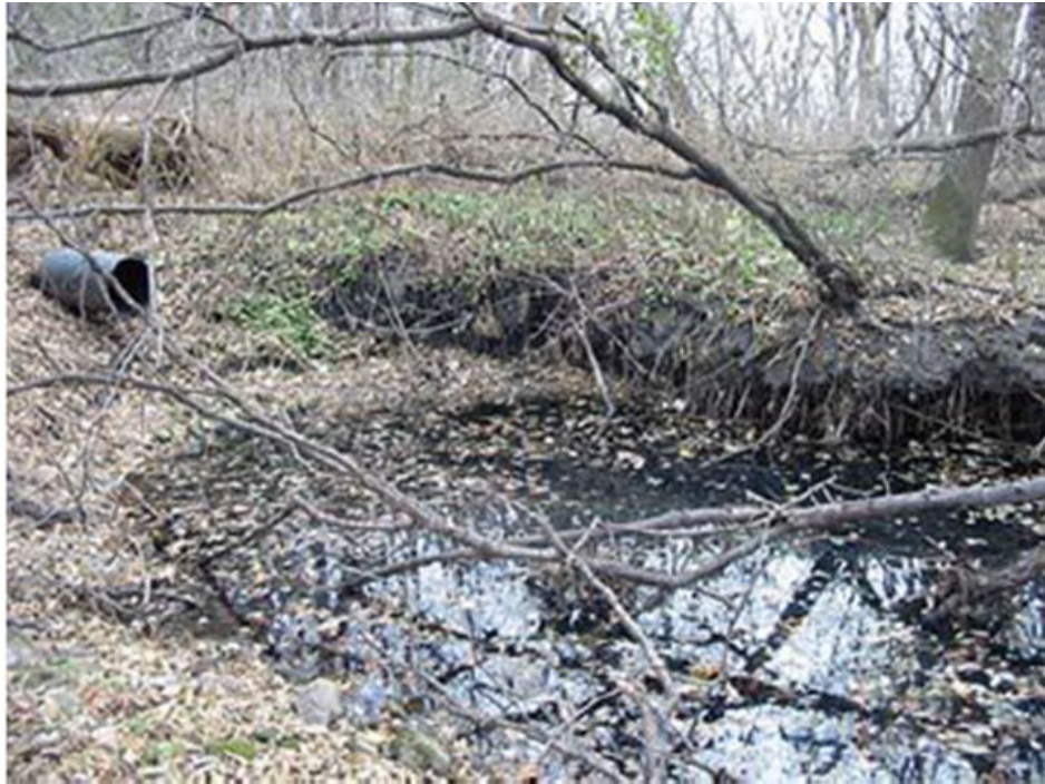
Figure 29. Photo from the 2008 Gully Inventory illustrating the pipe outfall and scour.
