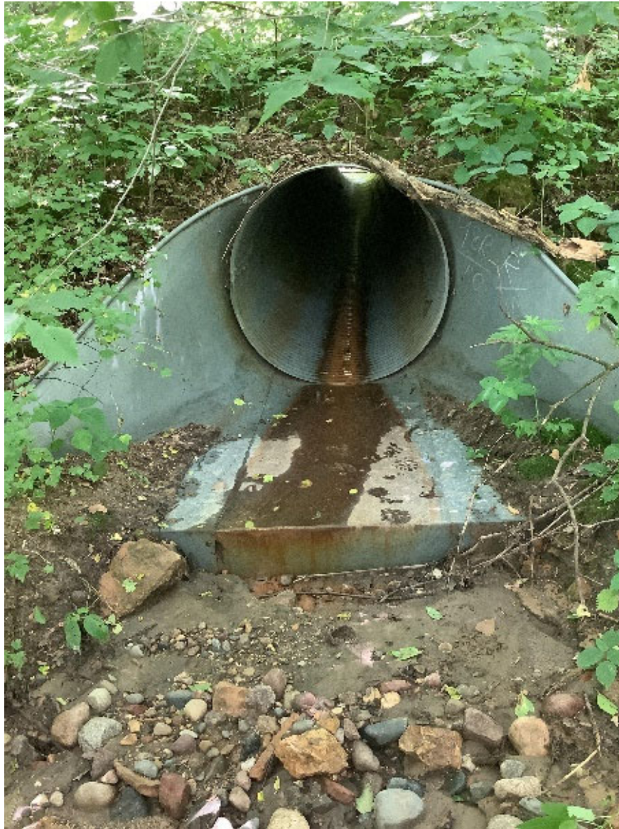
Figure 8. Example of a pipe outfall marked as “maybe” needing repairs.
