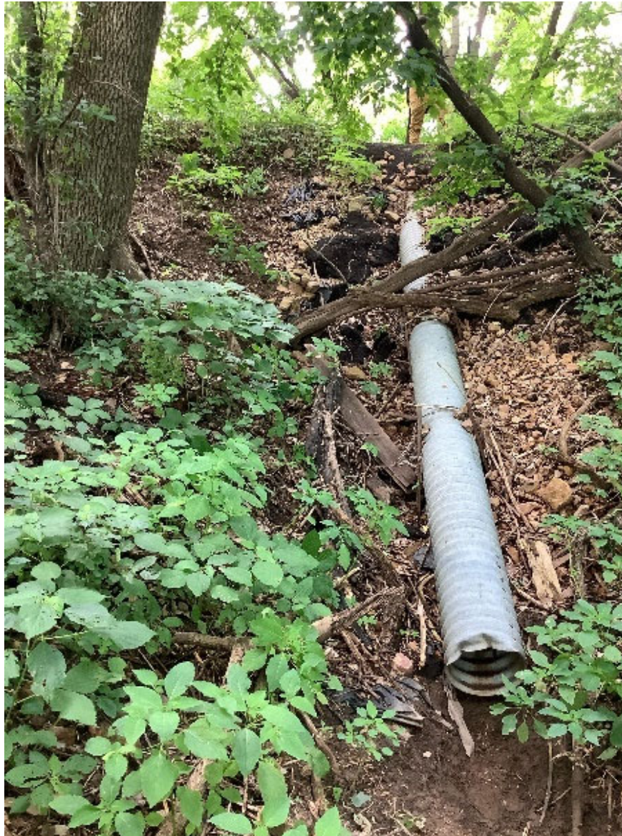
Figure 7. Example of a pipe outfall marked as needing immediate repair.
