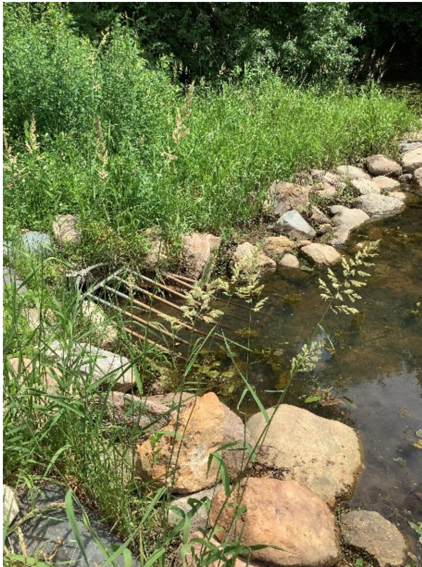
Figure 9. Example of a pipe rated as being stable and not in need of immediate repairs.
