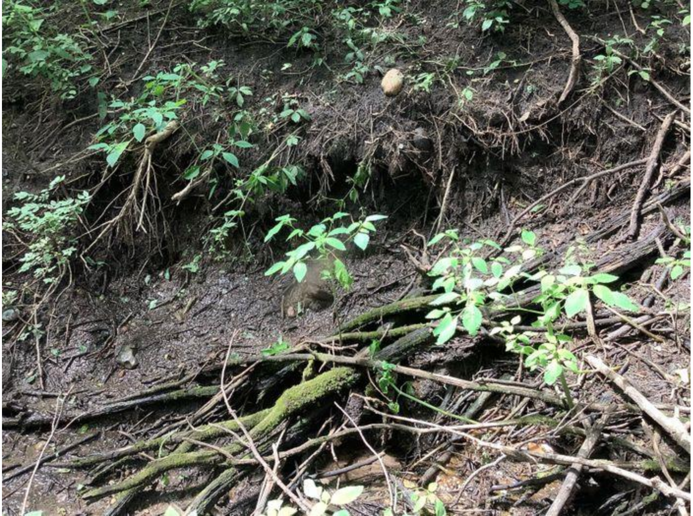
Side stream view from left bank looking at slumping and bare soil along right bank near headcut.
