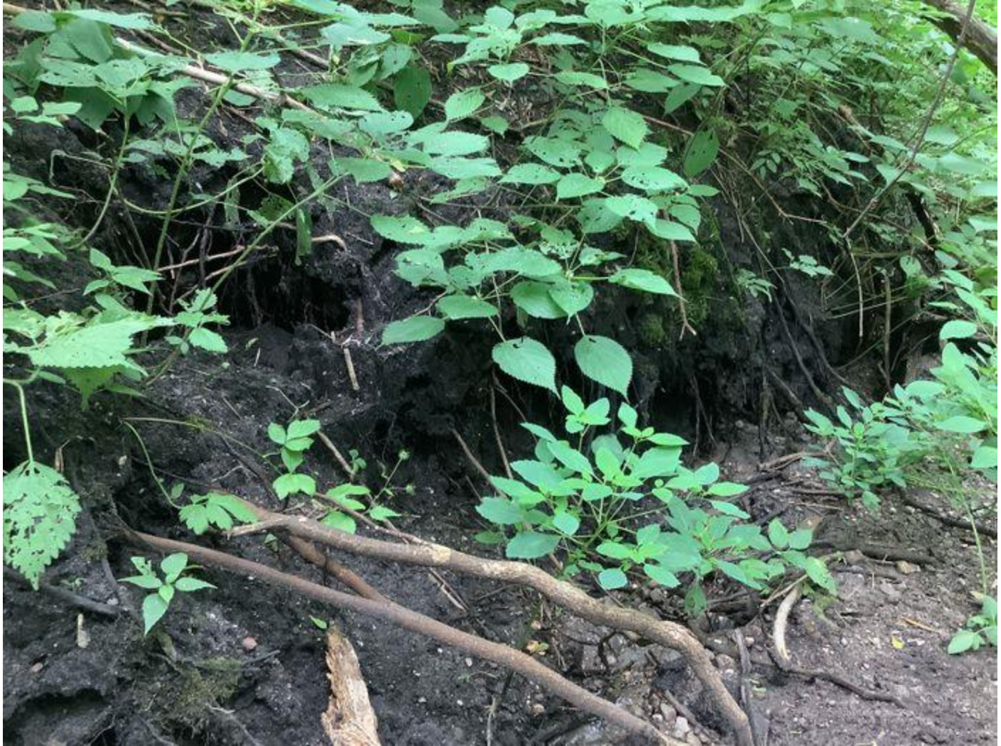
Looking d/s from right bank at a slump and severely overhanging left banks
