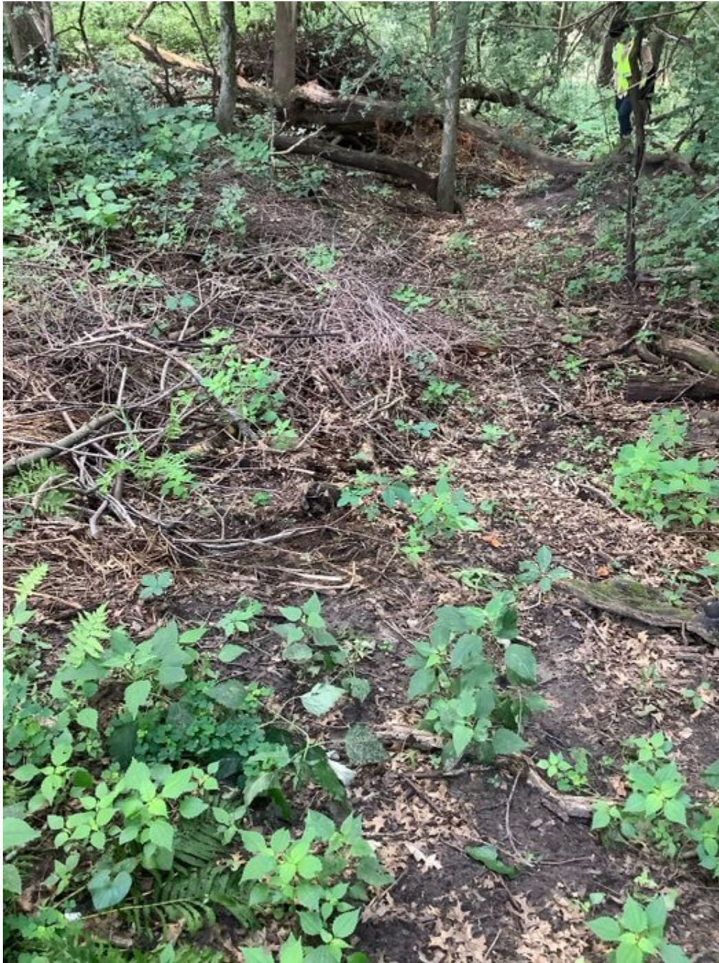
Downstream view from headcut looking at bare soil around headcut area but no signs of active slumping and tree debris piled in headcut channel.
