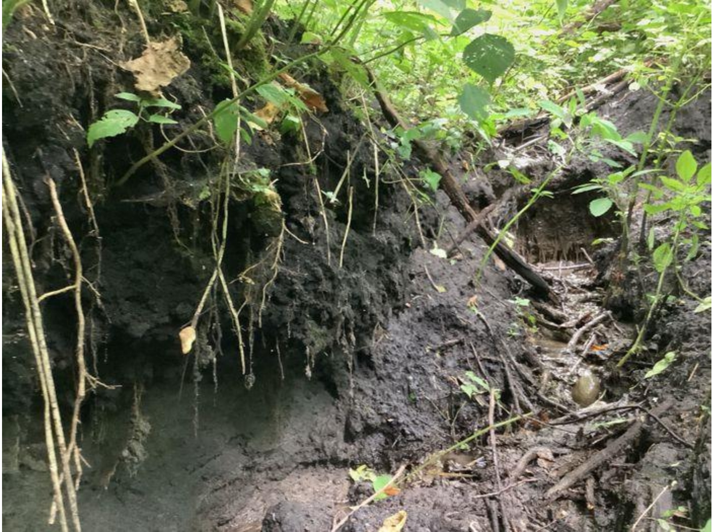
Looking u/s at overhanging right banks (d/s from initial slumping )
