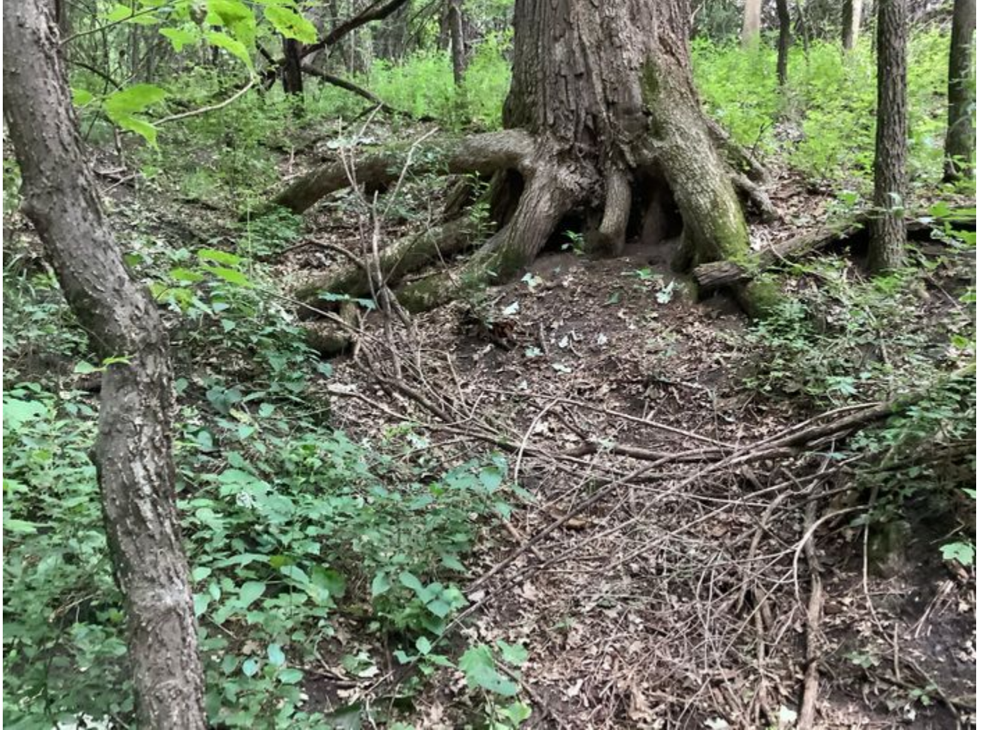
Looking u/s from gully toe towards left bank at exposed tree roots and bare soil
