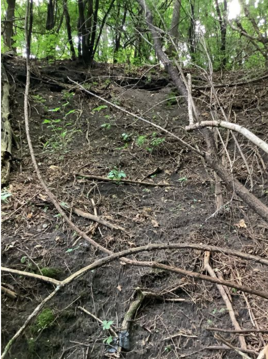
Looking u/s from gully bottom towards the headcut at the steep slopes and bare soil along the right bank
