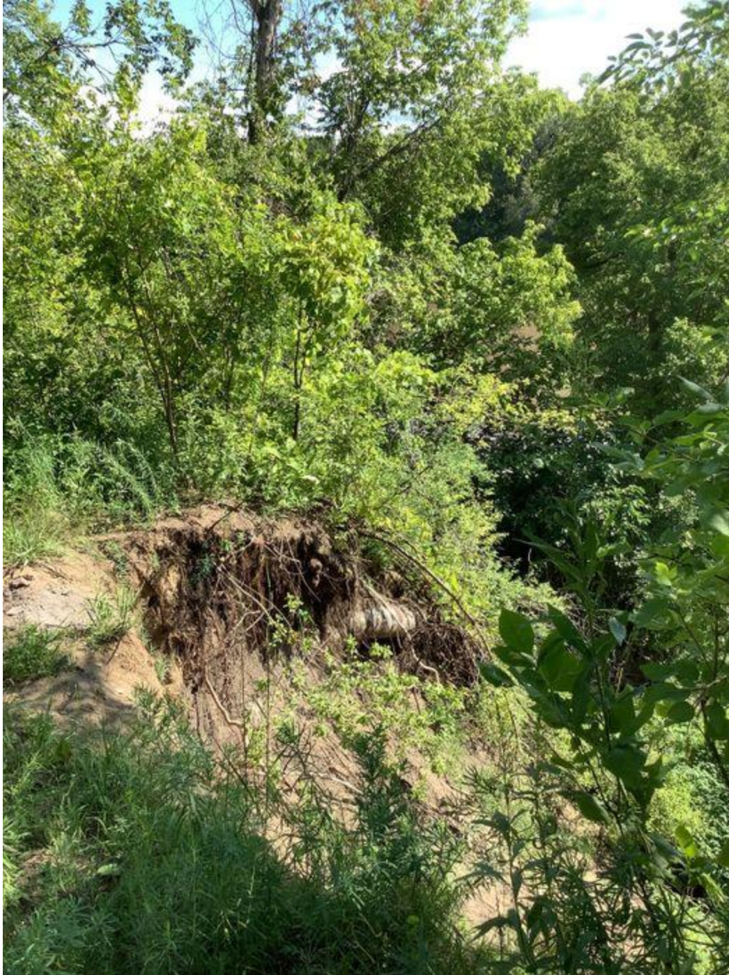
Pipe found along the left bank, but unable to assess due to steep slopes
