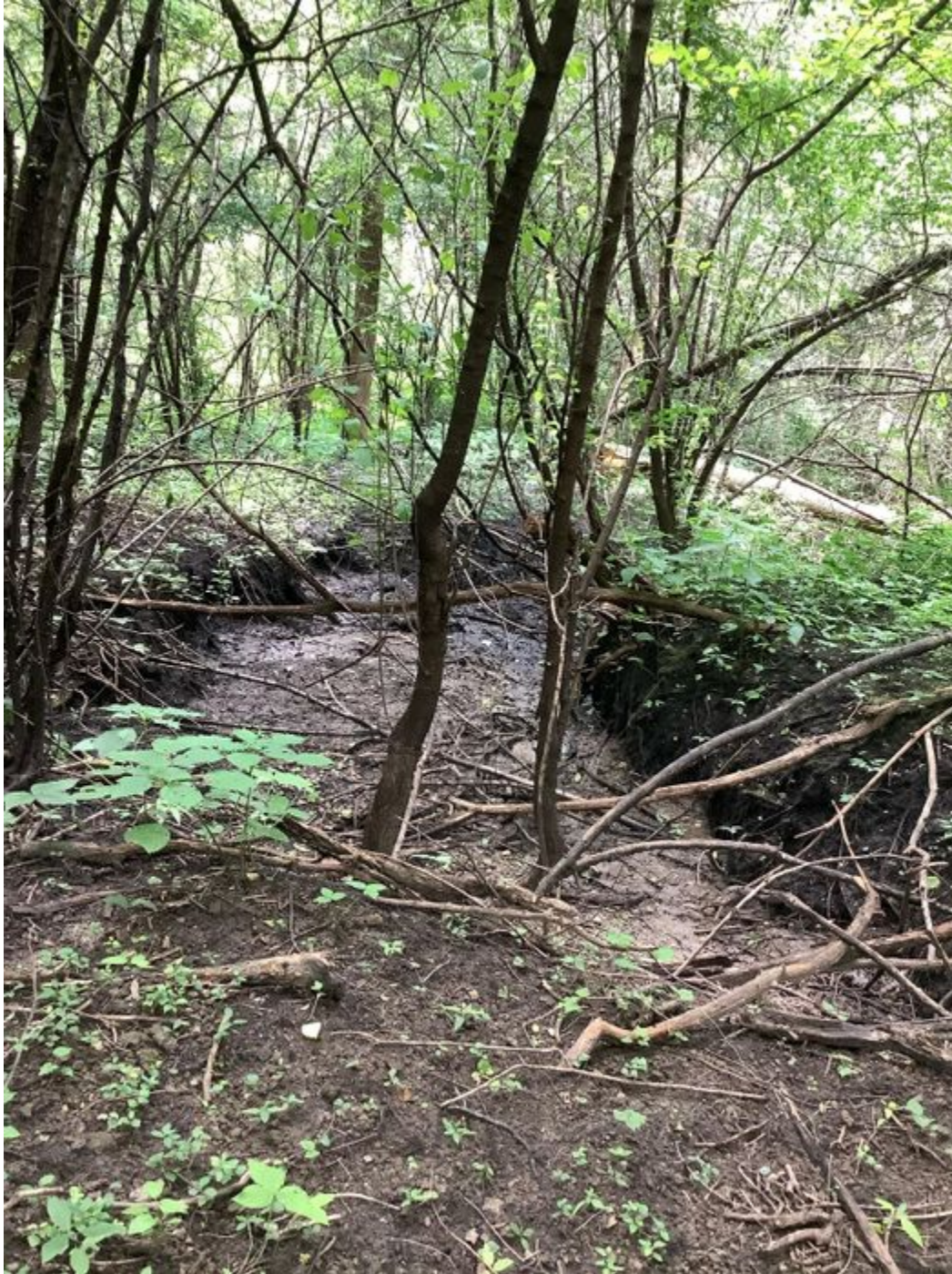
Downstream view from mid gully looking at overhang and slumping along both banks and a knick point close to the right bank.
