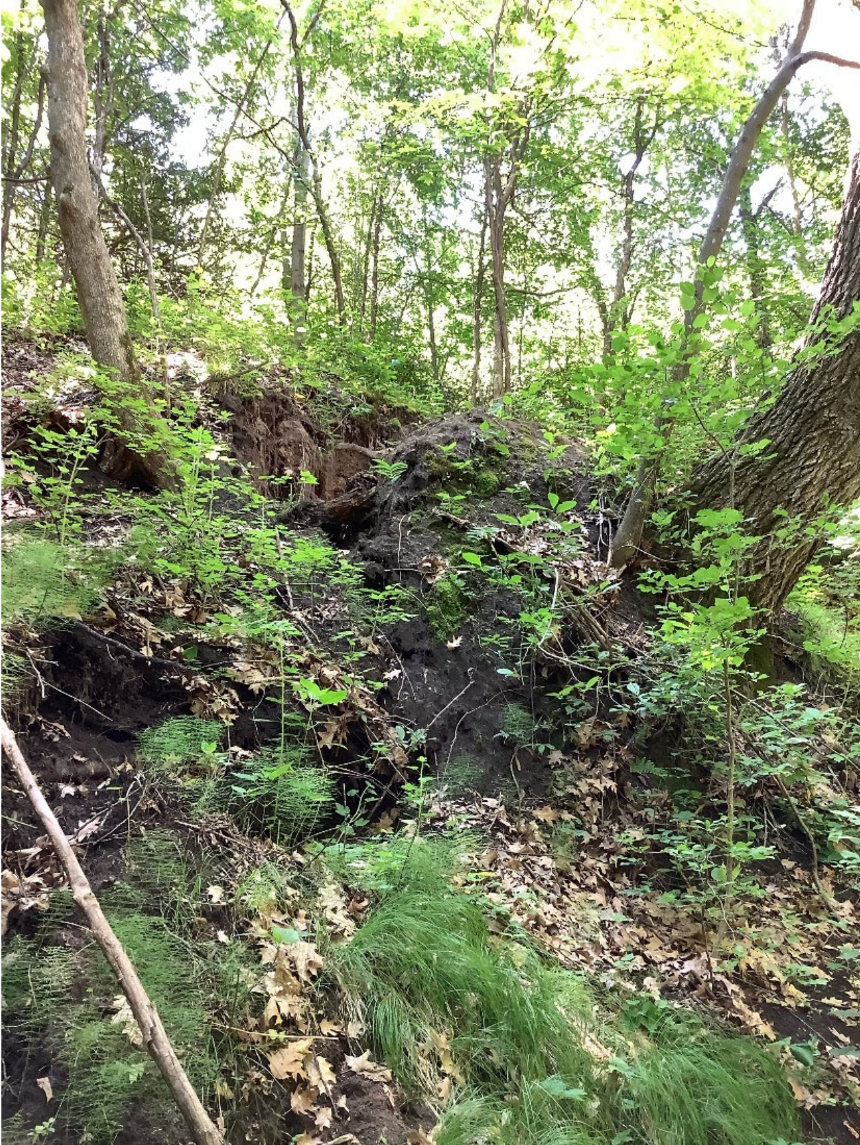
Figure 2. Looking upstream at left bank and actively leaning slump.
