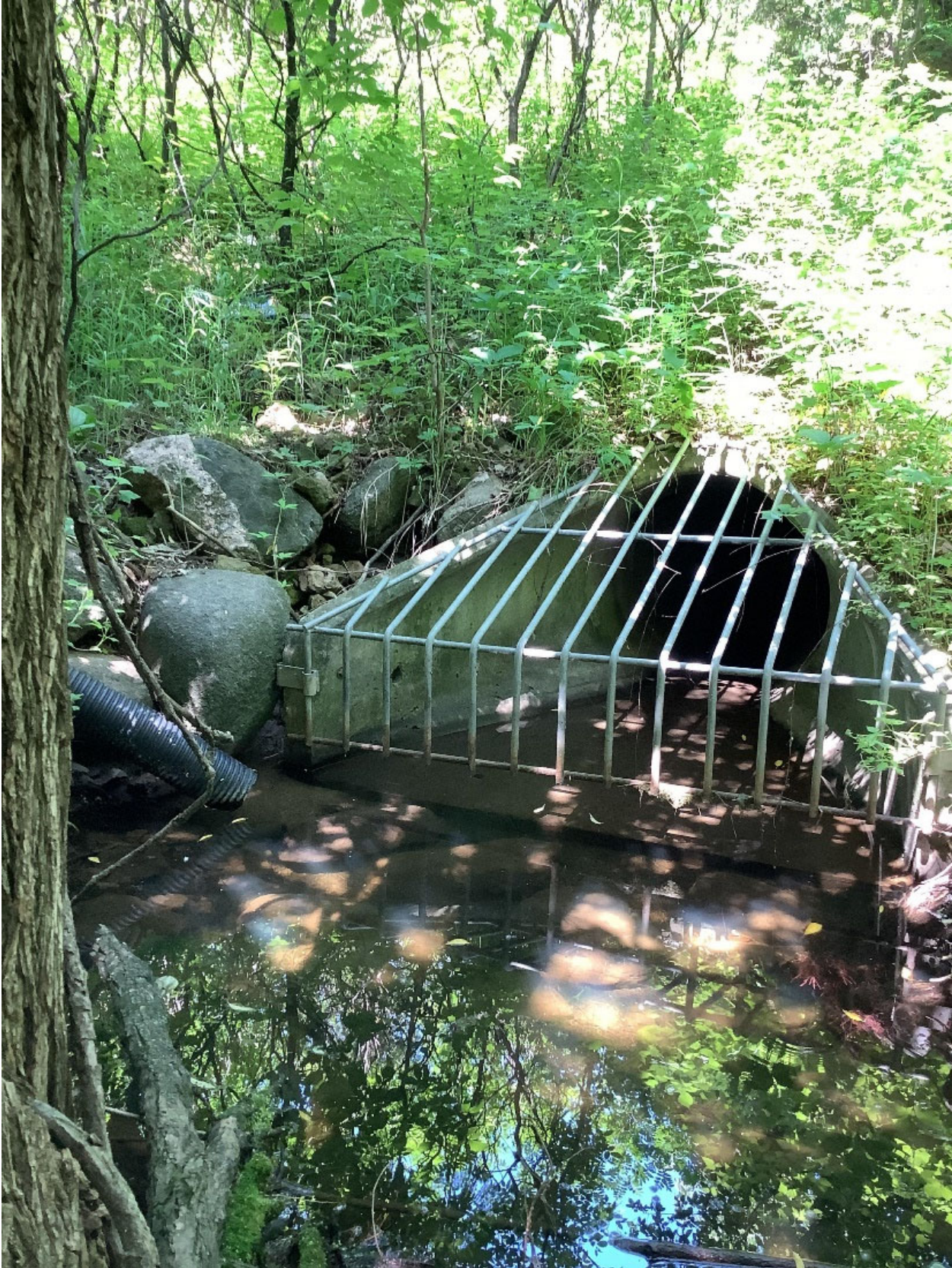
Figure 1. Scour on the right bank of the outlet pipe apron.
