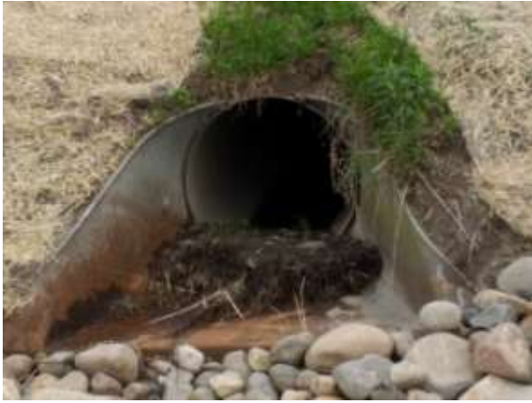
Secondary outfall to stabilized ravine. Pipe in under a service road to back of Riverland elevator
