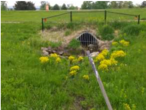
End of pipe from median of TH 101 - looking south from frontage road. Bike trail visible above outfall. This is a secondary drainage system draining to stabilized gully.
