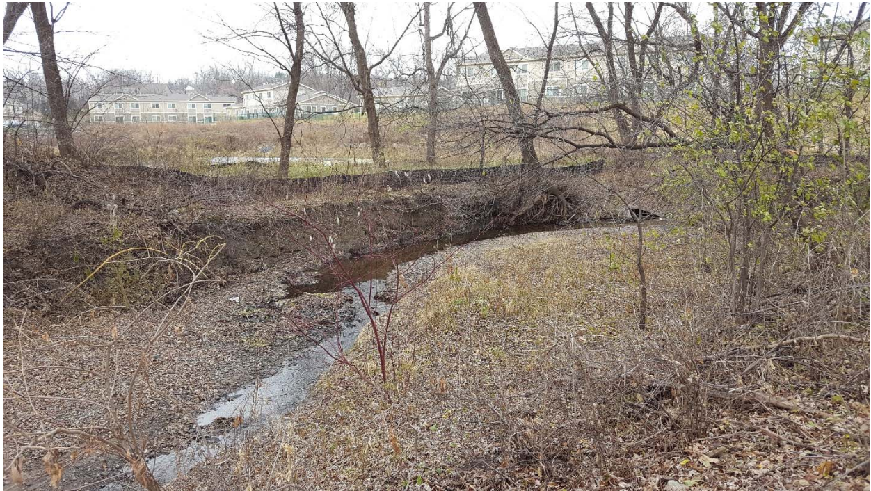
Photo 16: Site S5 – eroding bank and undercut trees
