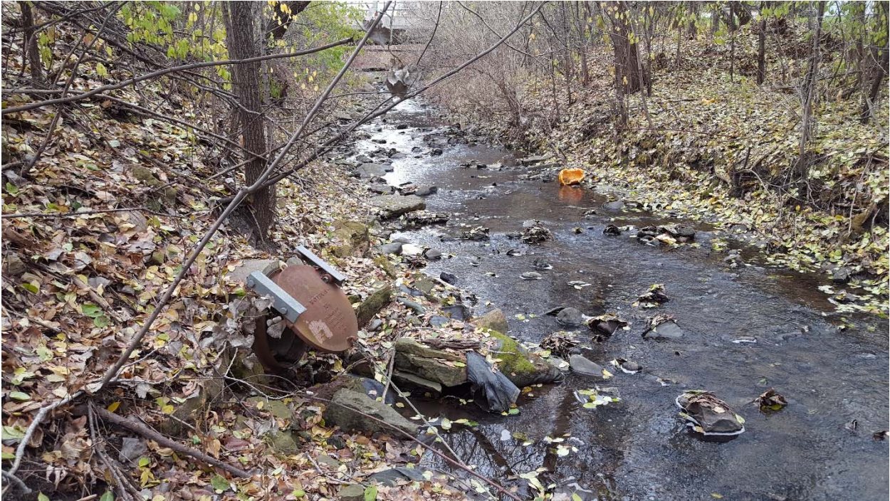
Photo 8: Site M11 – flap on RCP outlet and minor bank erosion
