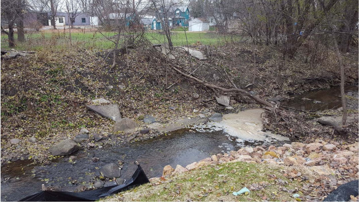
Photo 7: Site M10 – debris in channel downstream of site repaired by city of Chaska
