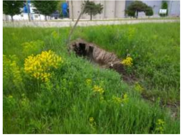
Other end of pipe under service road to back of Riverland elevator
