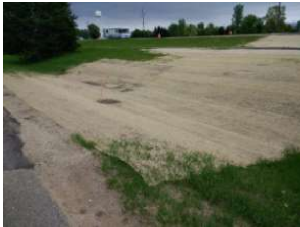
Looking east from frontage road in front of Murphy Landing Visitor Center. Erosion blanket covering excavation to install drainage from median of TH 101.
