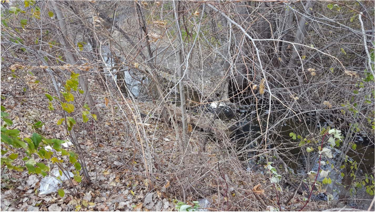
Photo 4: Site M7 – debris in channel causing blockage
