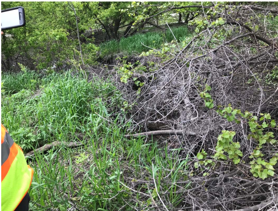
Photo 4. Eroding banks downstream of the spring
