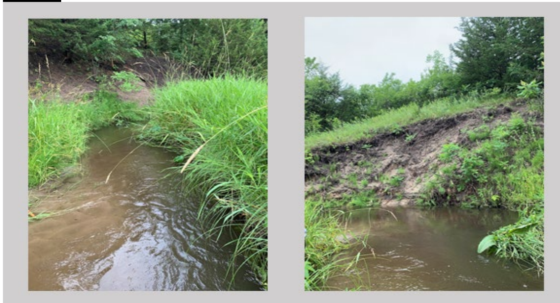
Figure E.5. Bank erosion and scouring at Point 18 on Eagle Creek East Branch. Kirsten Haus (June 2019).
