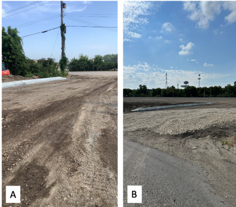
Figure 5. Fixed violation from the Former Knox site. A) Absent vehicle rock entrance/exit. B) Vehicle rock entrance/exit installed.
