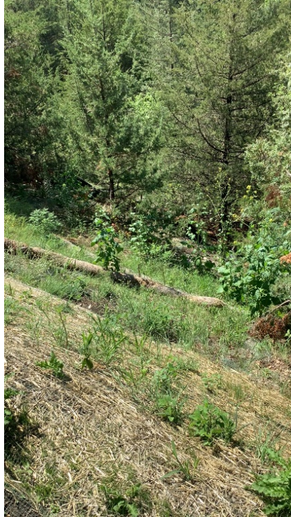
Figure 4. Engineering Hillside site with temporary BMPs present and lack of 70% vegetative cover.
