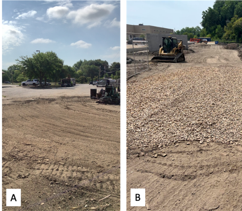
Figure 7. Fixed violation from the Chaska Tech Center site. A) Absent vehicle rock entrance/exit. B) Vehicle rock entrance/exit installed.
