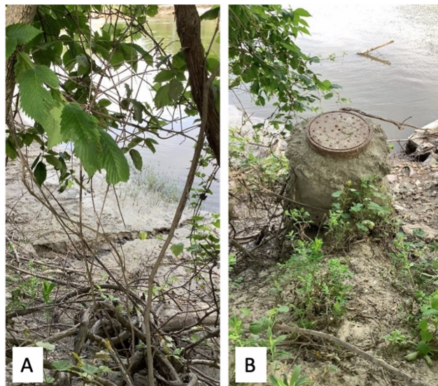
Figure 10. Photos of gully SHK10. A) Facing northwest looking down at gully. B) Image of structure that is surrounded by evident erosion.
