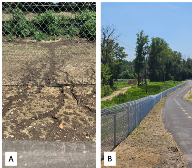
Figure 6. Fixed violation from the I35W Frontage Trail site. A) Rills running under fence. B) Repaired rills and laid hydromulch.
