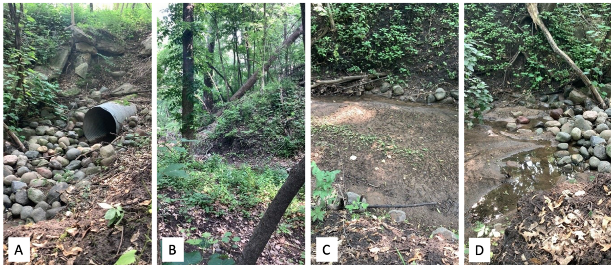
Figure 8. Photos of gully BVL62. A) Headcut with large pipe outfall and surrounding rip rap. B) Facing North at bank from the side of the headcut. C) Gully bottom condition. D) Image of water pooling at bottom of rip rap
