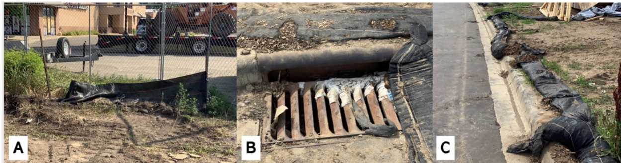
Figure 3. Example photos of violations found on-site. A) Damaged perimeter control. B) Dirty inlet protection. C) Damaged sediment logs.
