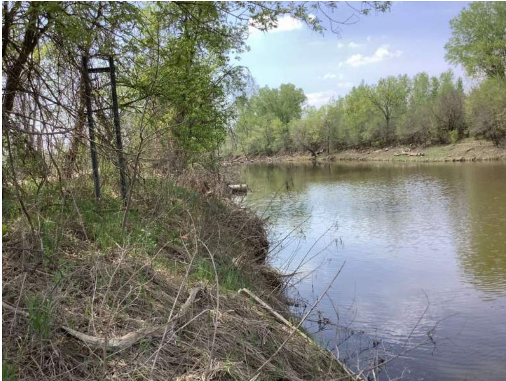
Photo 5 – View of Wetland A2, including a culvert connecting it to Wetland A3, facing south.
