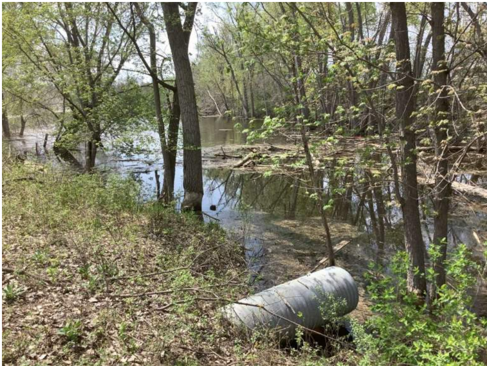
Photo 6 – View of Wetland A4, including a culvert connecting it to Wetland A2, facing south.
