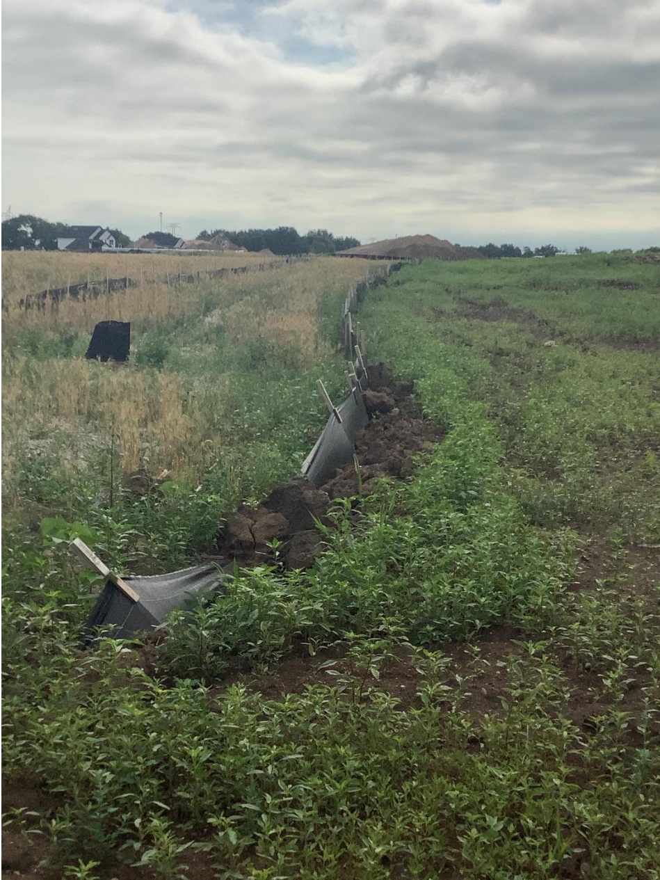
Figure 3. Overrun Silt Fence
