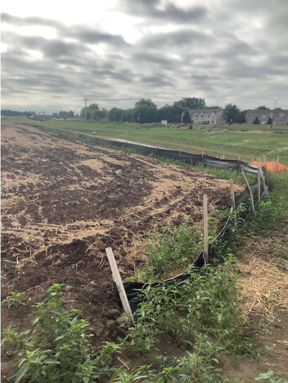
Figure 4. Fallen Silt Fence
