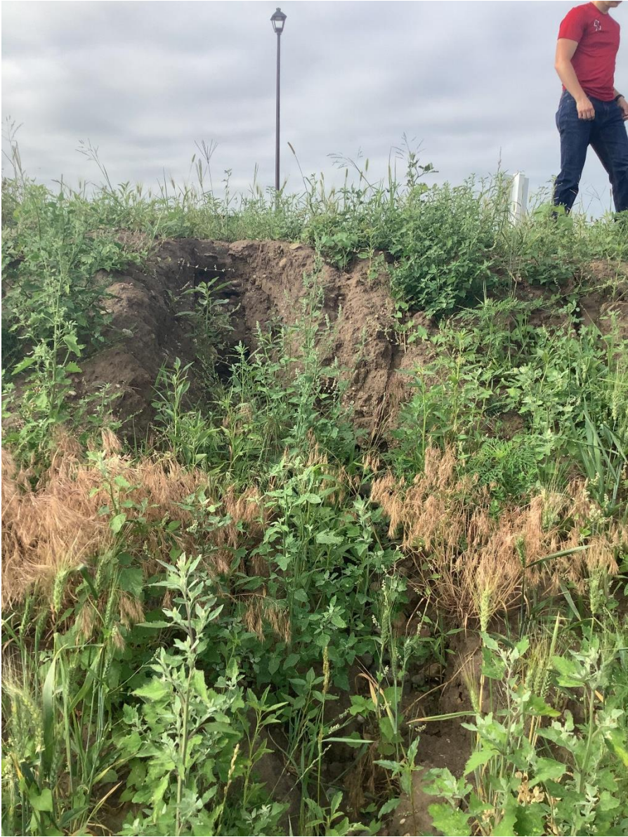
Figure 1. North Road Erosion
