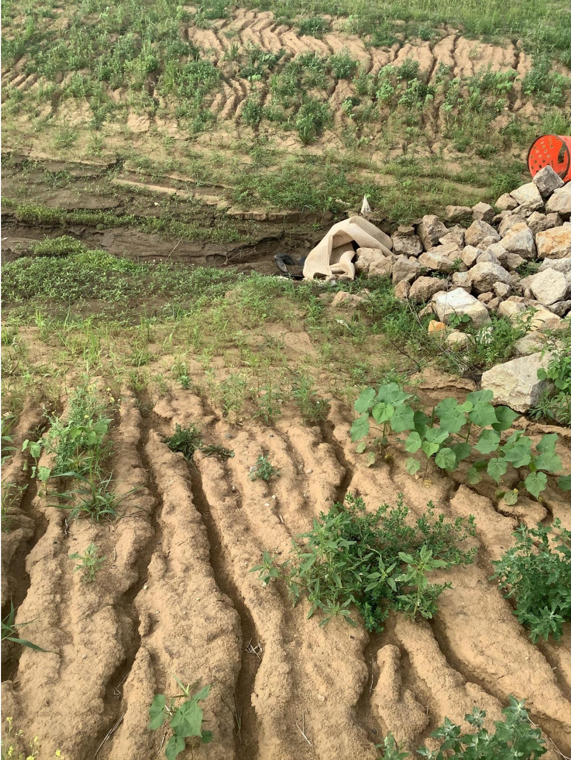
Figure 5. Rills on the Infiltration Basin Walls
