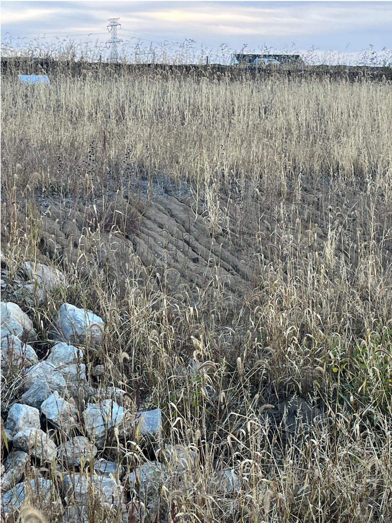
Figure 6. Remaining Rills on Infiltration Basin 10/12/2022
