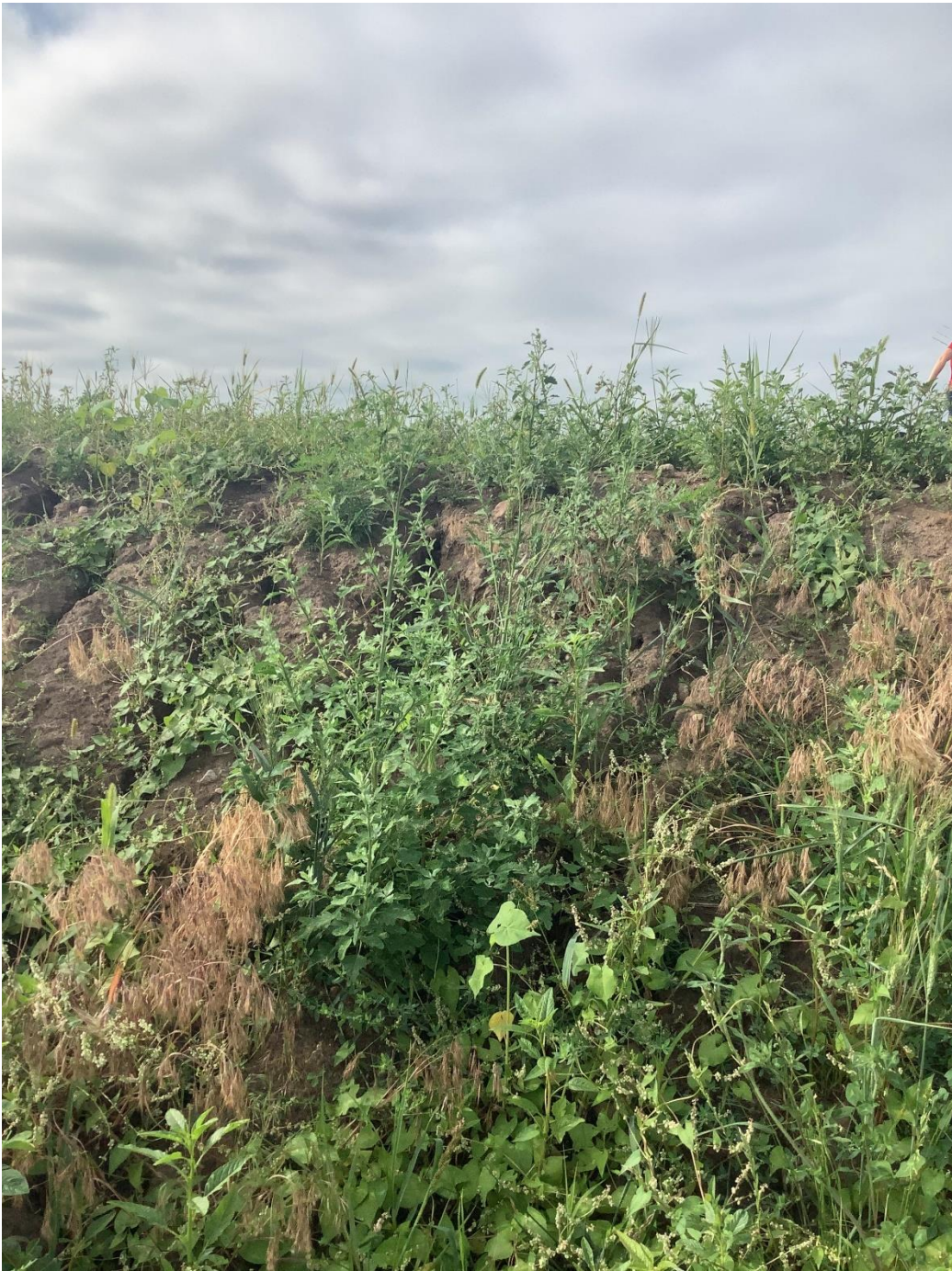
Figure 2. Further North Road Erosion
