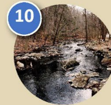
10 City of Burnsville Willow Creek Ravine Stabilization (see page 7)
