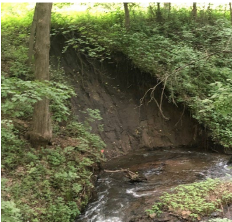
Above failed bank on Riley Creek near Dell Road, 2020.
