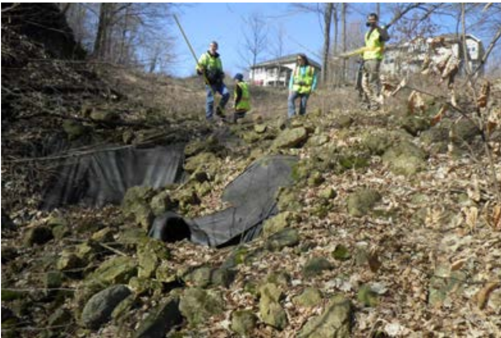
Photo 2. Site D3. Failing riprap downstream of storm sewer outfall (photo is looking upstream)
