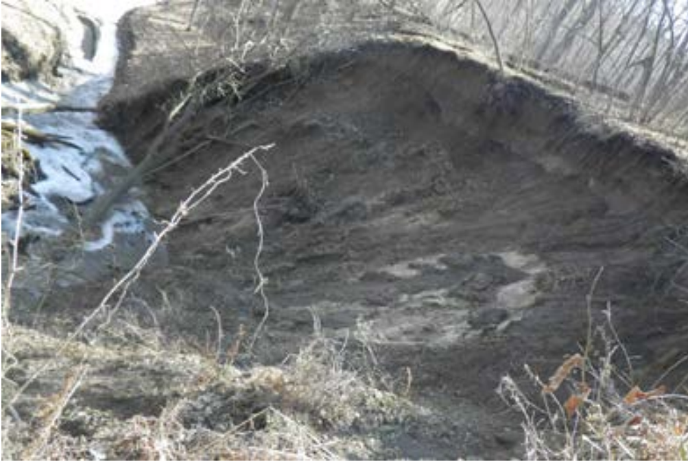
Photo 9. Reach E2. Severe scarp erosion in left overbank
