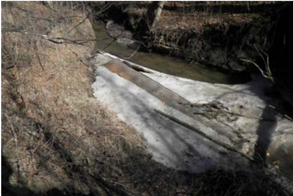
Photo 20. Reach E3. Abandoned pipe in stream channel
