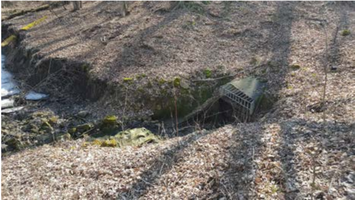
Photo 15. Reach E3. Perched culvert outfall in left overbank
