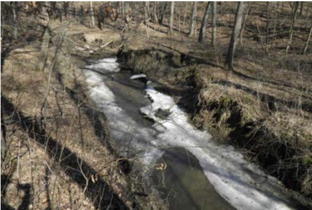
Photo 14. Reach E3. Channel degradation and bank erosion (looking downstream)
