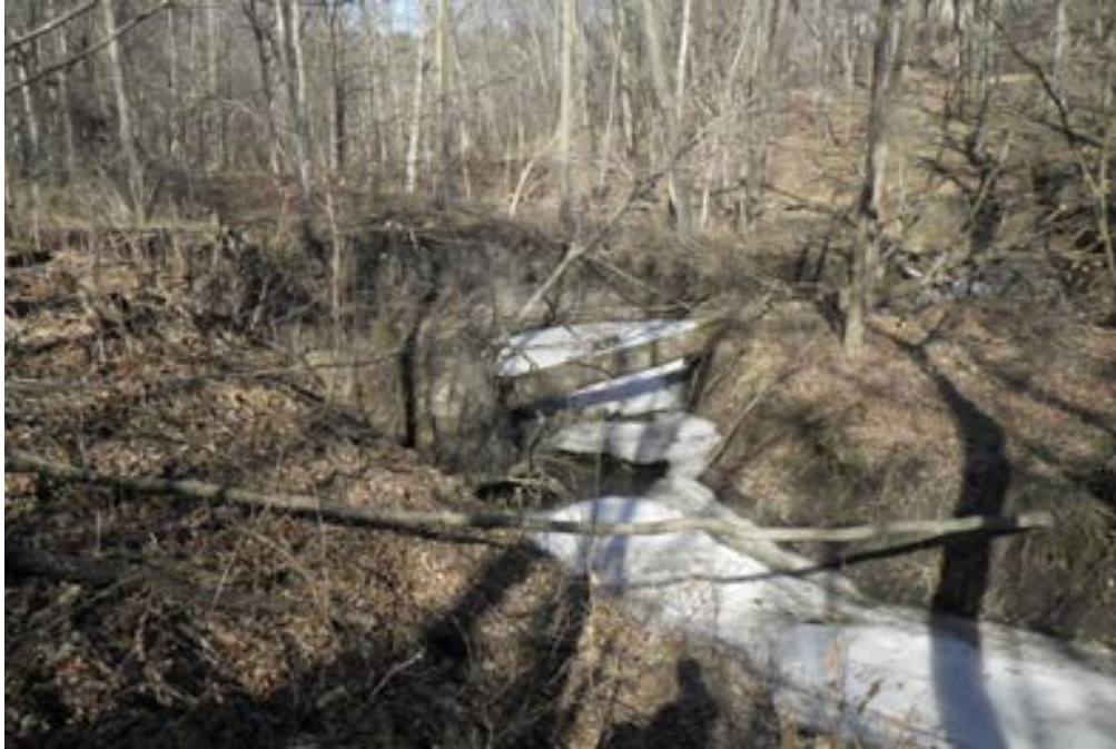
Photo 21. Reach E3. Channel degradation and bank erosion (looking downstream)
