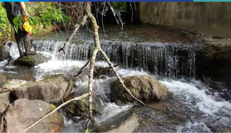
Scouring on the downstream side of Flying Cloud Drive is representative of active erosion in Riley Creek
