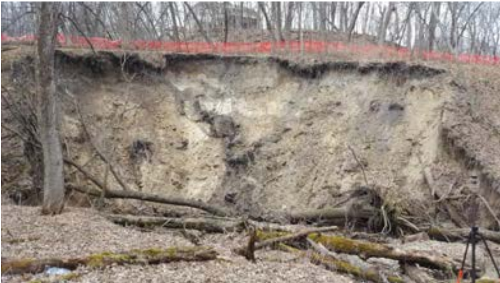
Photo 10. Reach E2. Severe scarp erosion in left overbank
