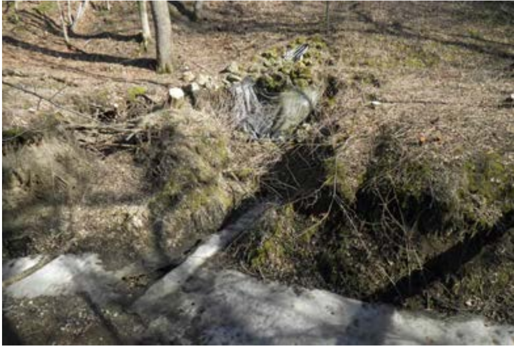
Photo 17. Reach E3. Perched culvert outfall in right overbank
